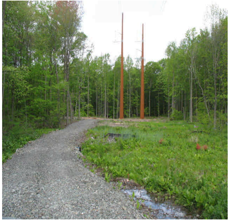
View of wetland crossing from the contractor yard. Re-growth of vegetative cover is well underway.
