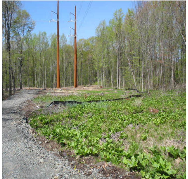
Stock piles and pad were removed/reclaimed at the CSC approved pull site. Controls will remain until final stabilization with vegetative cover occurs.
