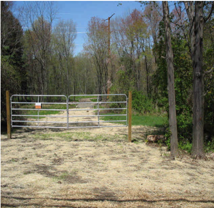
Water levels remain high at the drainage bisected by the new access road. It appears a culvert will be necessary to maintain flow/hydrology in this area. Contractors have evaluated this area and improvements will likely need to wait until a low flow period to minimize additional disturbance.
