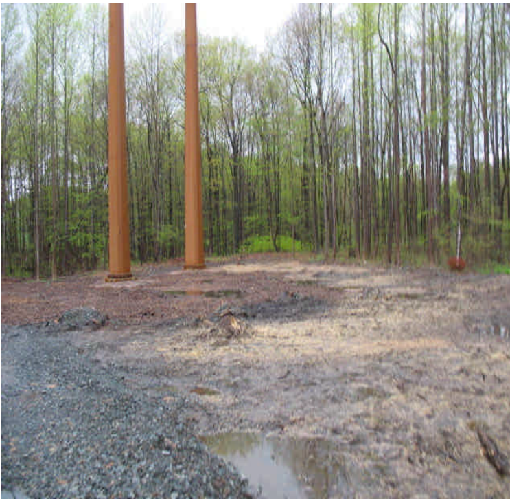
Small stockpiles have been removed from the upland adjacent to the contractor yard.
