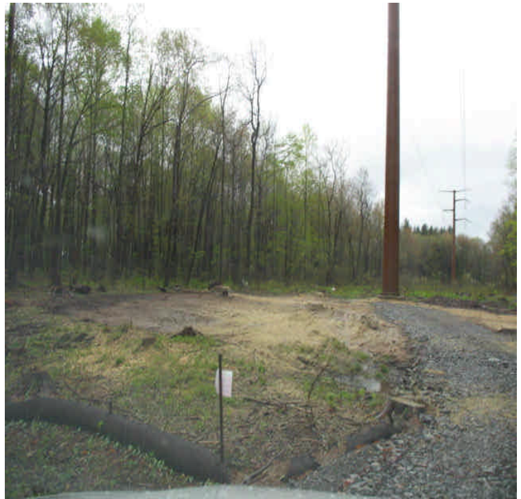
Stone pad was removed, graded and hay and seed applied at structure #24531.
