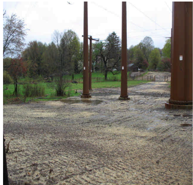
Timber mat removal and final grading from Rte 17 to Little Ln is complete. Monitor for final stabilization with vegetative cover.
