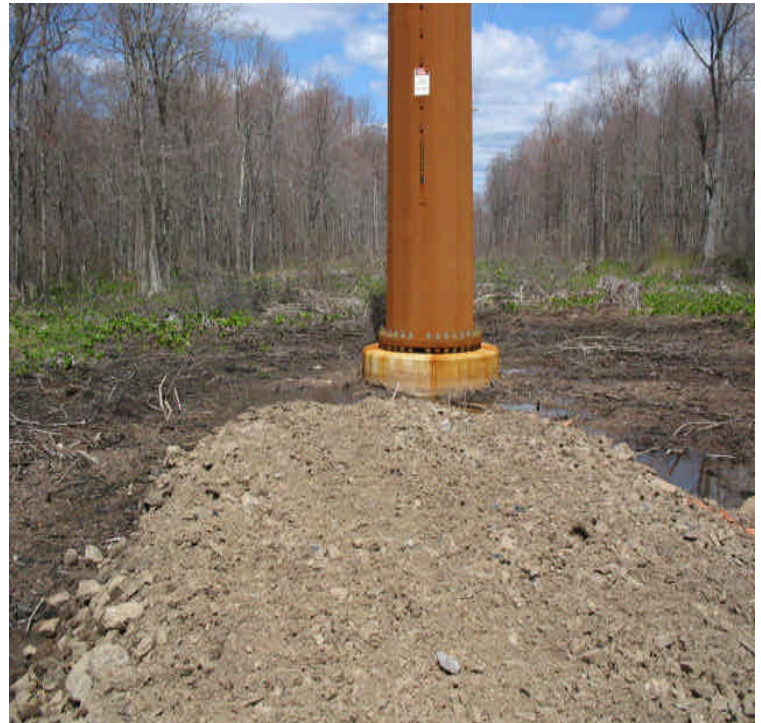
End of the new access road at structure #24580. Exposed area of soils noted from timber mat removal. Amphibians were noted within a small pool at the end of the access road near the new structure. Final stabilization/restoration still needed here.
