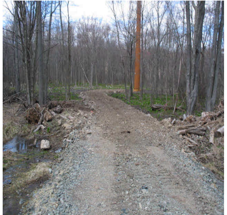
New stone access road installed west off Rte 17 between the receiving yard and north of Little Lane, in order to maintain access to structure #24580.
