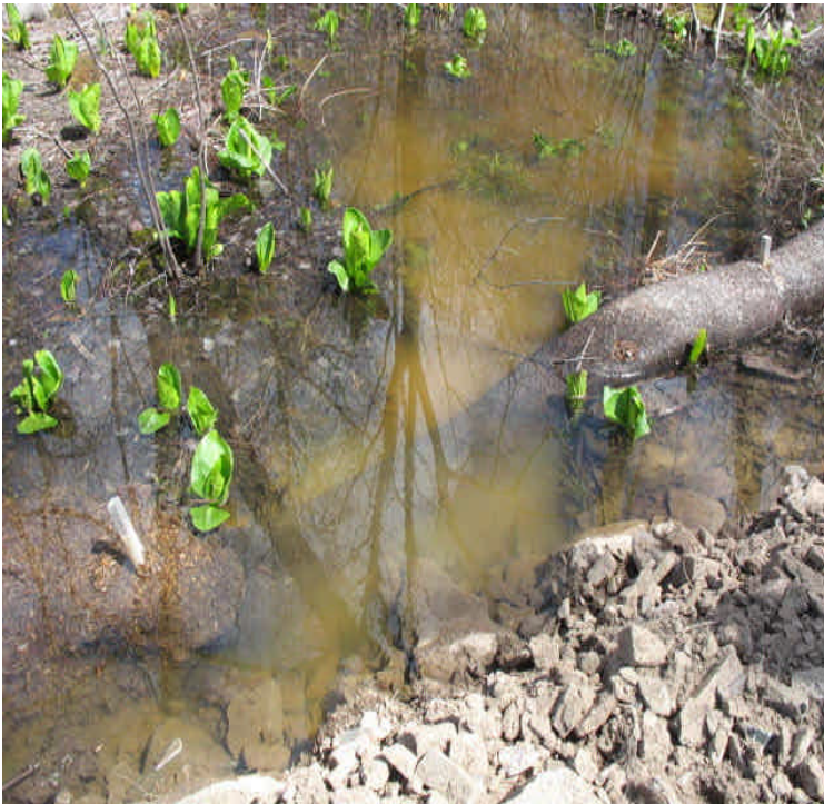
Small flooded channel bisected by the new access road. Some turbid water and sediment were noted from the access road installation. Flow and hydrology will need to be maintained in this area with use of a culvert.
