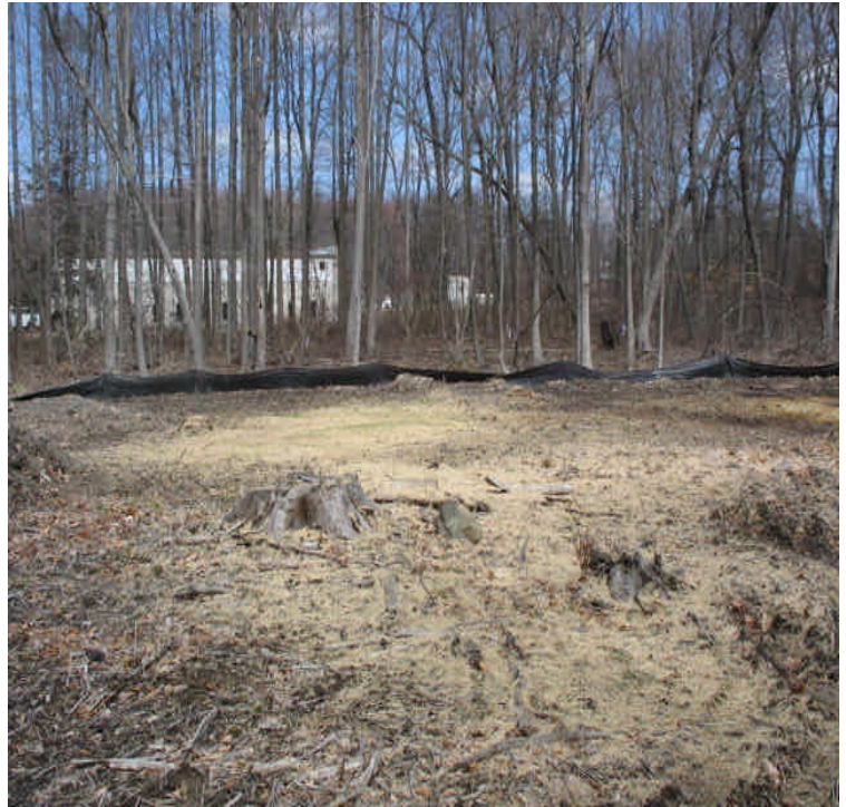
View of the CSC approved line-pulling area. Stone was pulled back from wetlands and stockpiled. Controls remain in place along with hay/seed
