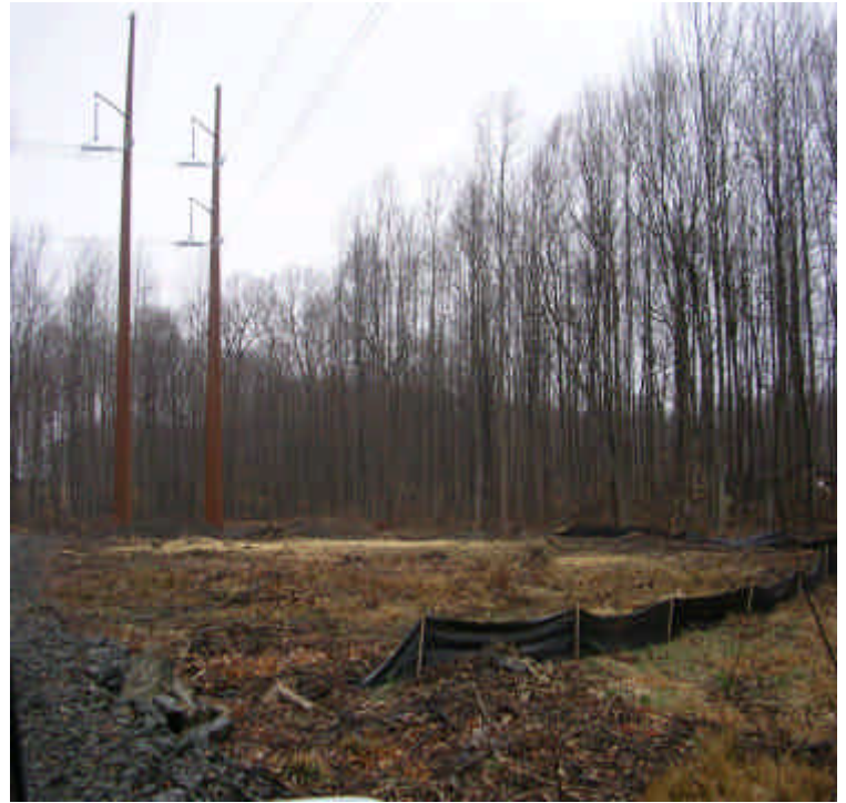
CSC approved line-pulling area. Stone was pulled back from wetland and stockpiled. Controls remain in place along with hay/seed.
