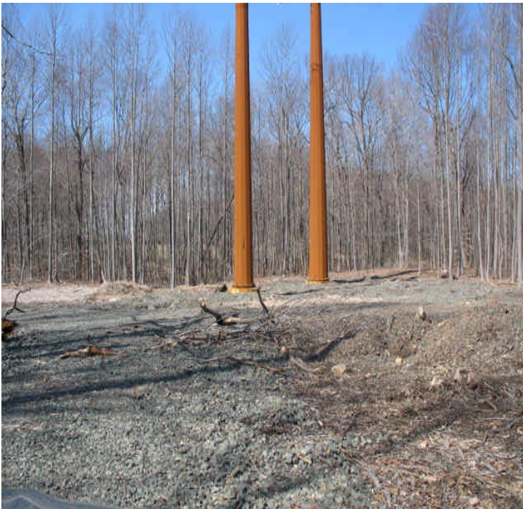
Final reclamation is still needed from the turn in the ROW at the receiving yard to Little Ln.
