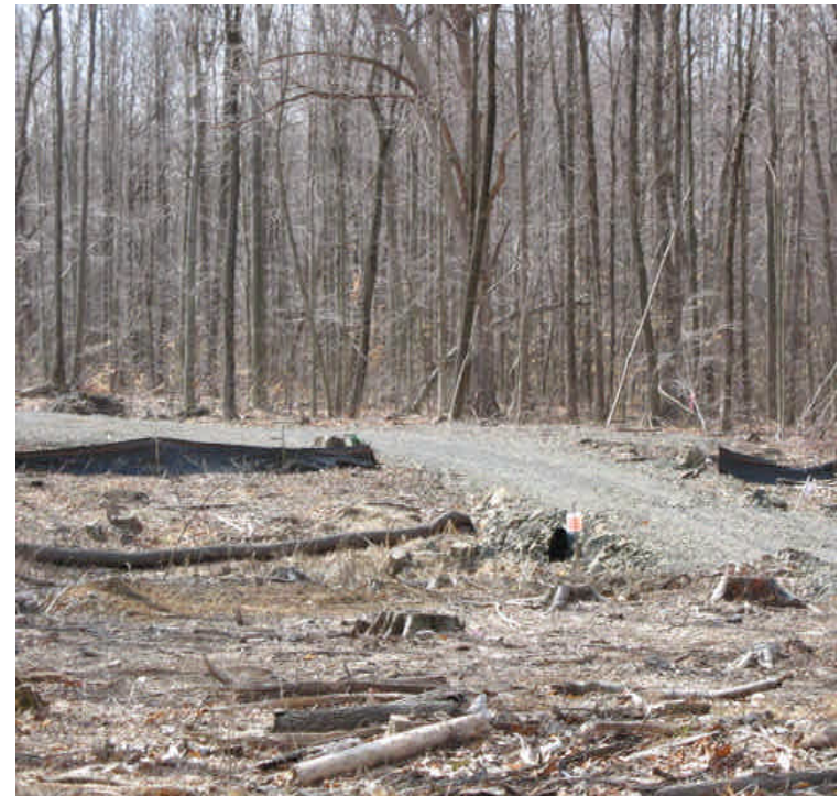
View of the stream crossing on the access road from the receiving yard. Controls are in place.
