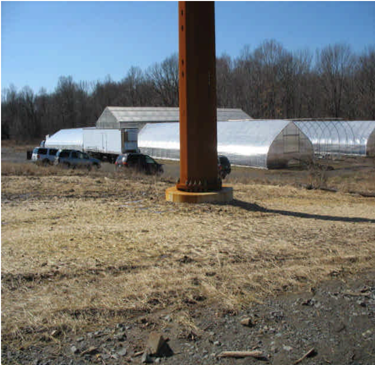
Hay and mulch were applied at a reclaimed pad site within the the receiving yard . Fiber roll controls are installed downgradient from the exposed area.
