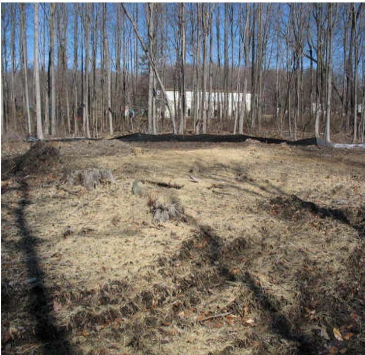
Hay and seed were applied over the reclaimed pull site. Silt fence was installed adjacent to the wetland.
