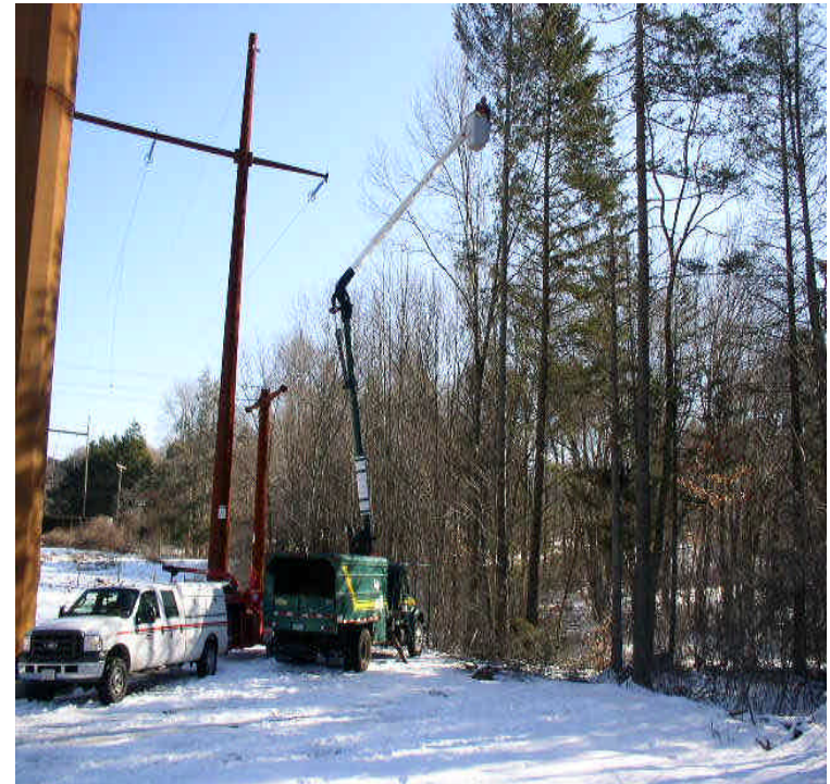
Little Lane: Minor tree trimming underway at the edge of the ROW.
