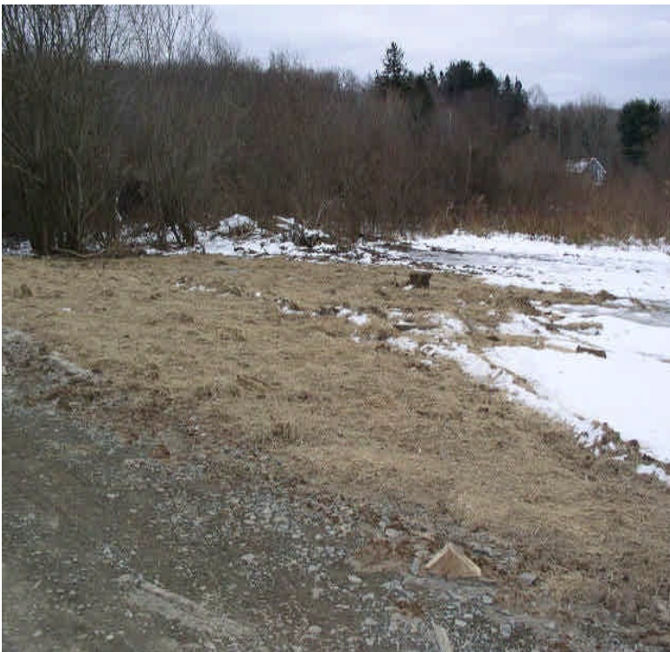
Contractor receiving yard. An old pad and storage site was graded and temporarily stabilized with hay mulch and seed.
