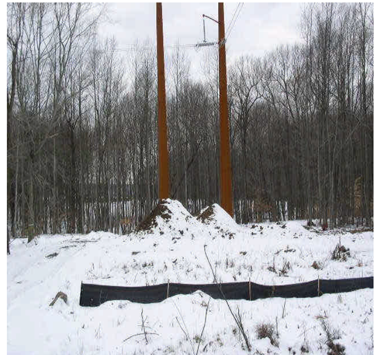
Soil stockpiles remain near the edge of the wetlands near the receiving yard. Ensure that controls are in place and stockpiles are not stored within 100 feet of wetlands where feasible.
