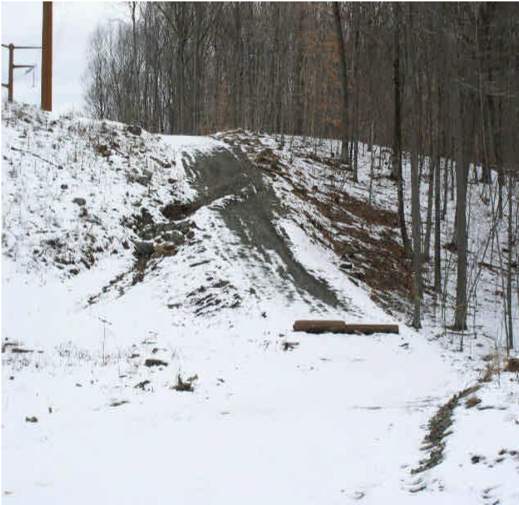
The slope off the Black Walnut Dr. entrance has a drainage ditch/water bar to divert run-off and an old wooden pole to prevent vehicles from driving over and damaging controls.
