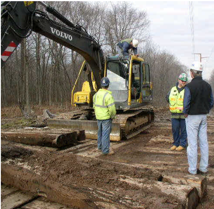
Timber mat removal underway within the wetlands off Rte 17 near Little Ln. Encourage vegetative cover as soon as feasible and provide mulch in adjacent upland areas.
