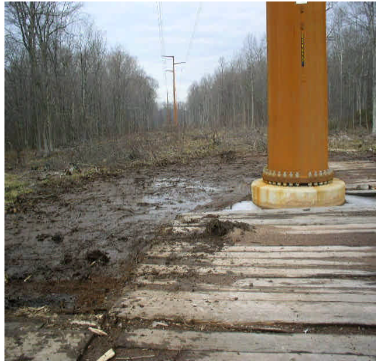
Disturbed area where pads were recently removed within the wetland off Rte 17 near Little Ln. Carefully restore contours upon completion of pad removal and encourage vegetative cover as soon as feasible.
