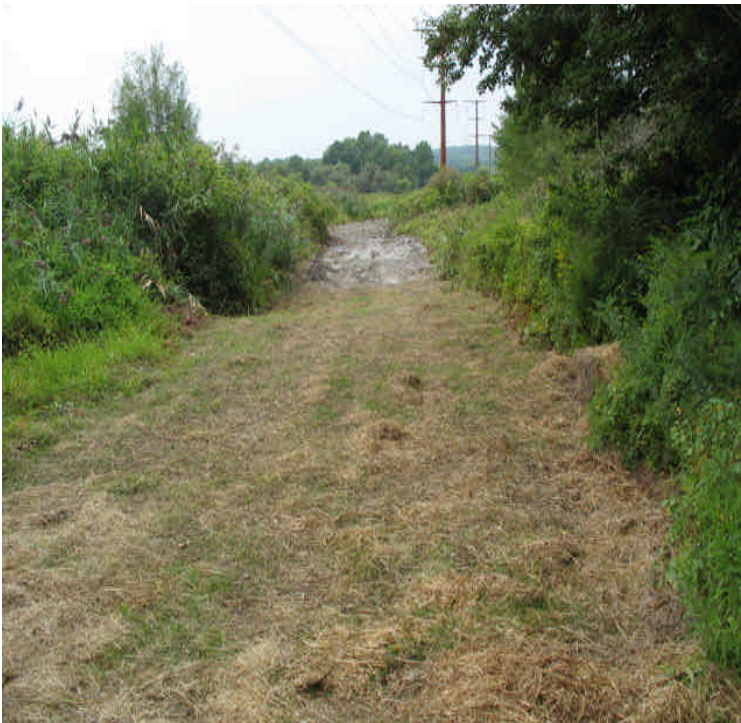
Durham Rd: Final restoration complete within Durham Meadows. Check/add controls and monitor the area until stable. Areas out of the standing water were mulched and seeded.
