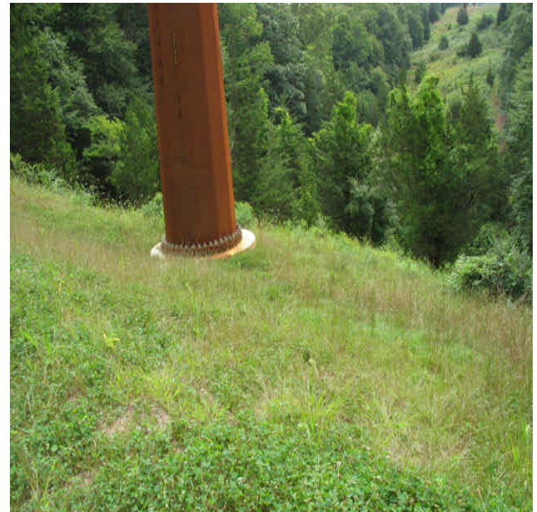
Black Walnut Dr: Vegetation continues to grow along the slopes upgradient from Ball Brook. This segment is stable with at least 70% cover.
