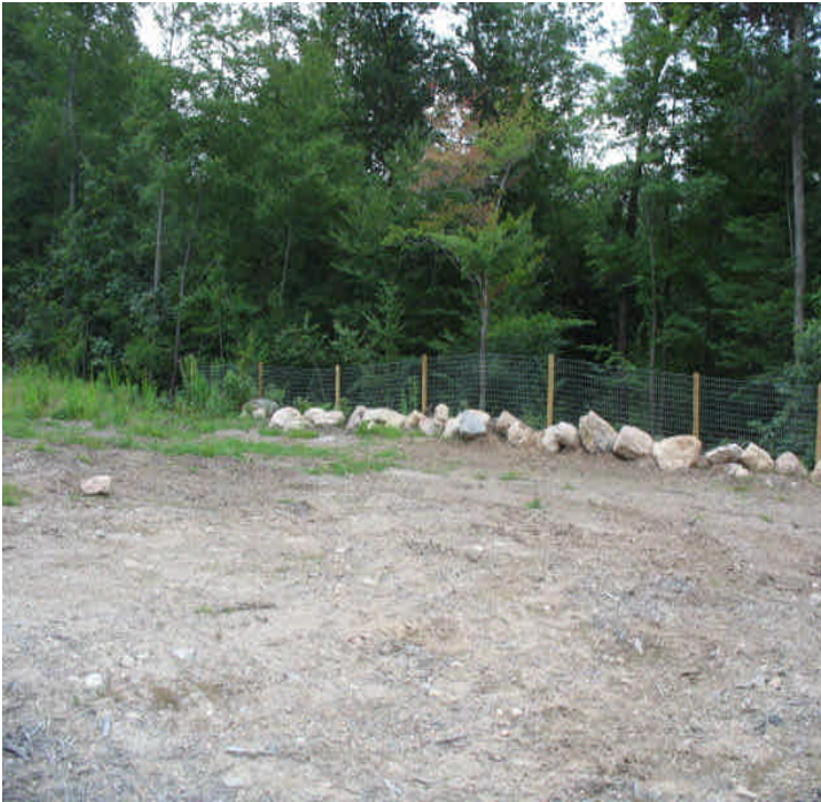
Rte 9: View of restoration of a hiking path along the ROW between Rte 9 and Scovill SS.
