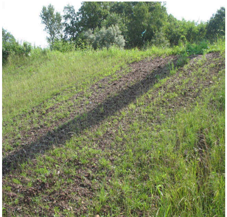
E. Meriden SS: Sparse vegetative growth/cover was noted on the slope downgradient of the substation but the area is fairly small.
