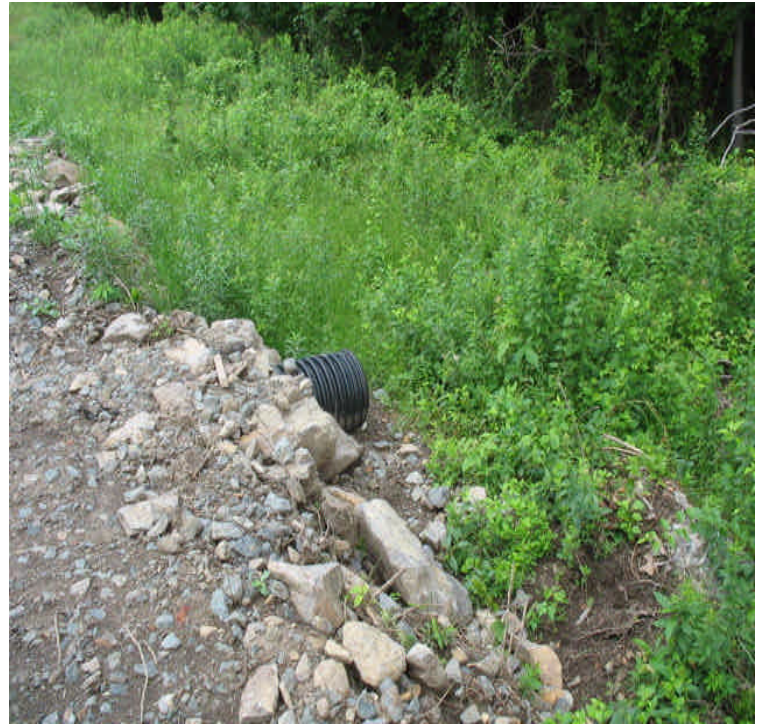
Haddam Quarter Rd: View of the culvert at the saturated crossing. This area is currently dry and good vegetative growth was noted.
