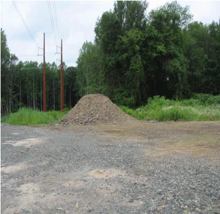
Contractor Yard: Even though it has been temporarily stabilized with seed and mulch and controls are in place, the stockpile located upgradient from the wetlands at 1B should be moved.
