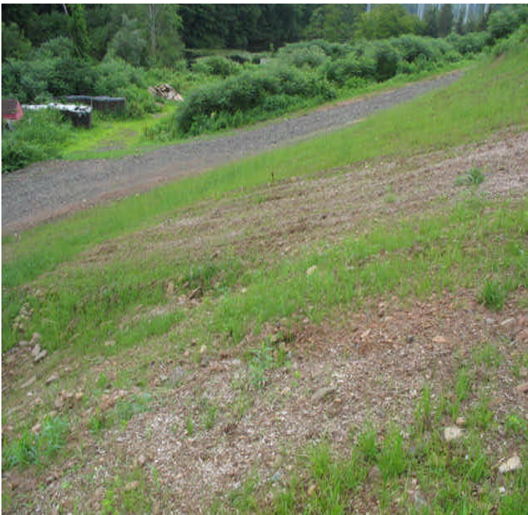
E. Meriden SS: Vegetative growth along the slope below the switching station is sparse and may need additional seed under more favorable conditions.
