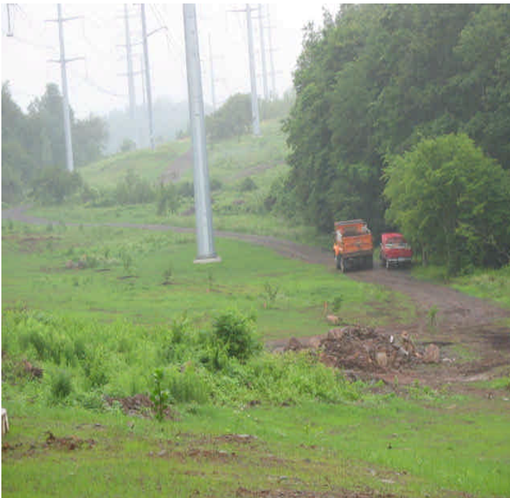
E Meriden SS: Crews were planting shrubs along the ROW. Grass cover was noted in recently seeded areas.
