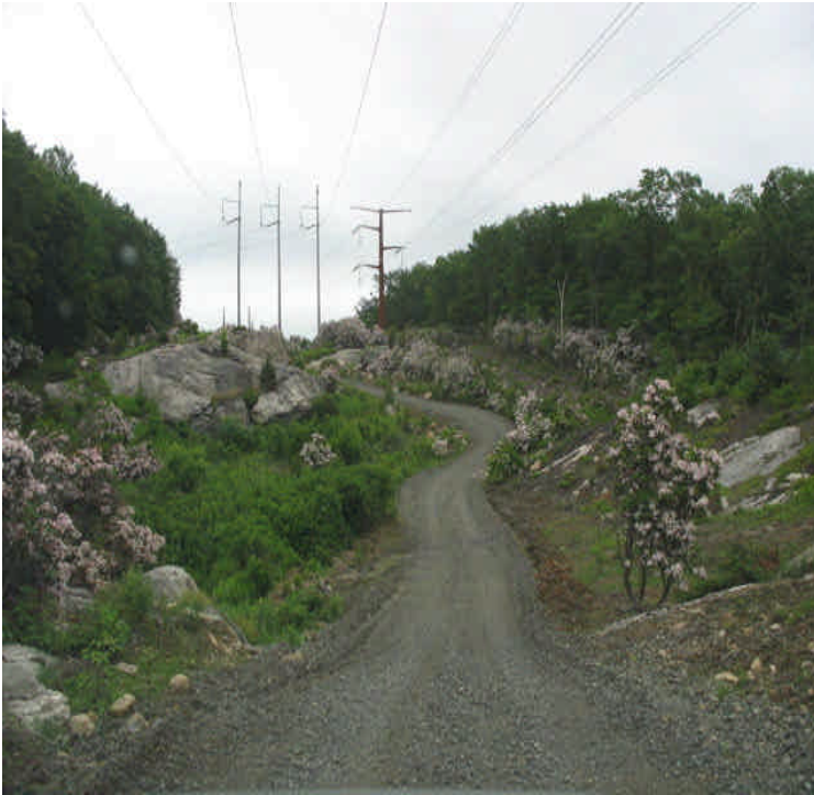
Scovill SS: View of vegetative growth along the access road near the switching station. Mountain laurels were retained as appropriate low growth, woody species.
