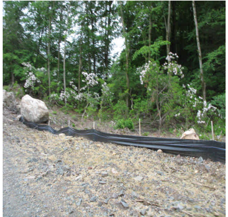
Saybrook Road: Final restoration complete, controls remain from Saybrook to Scovill. When adjacent areas stabilize, silt fence will have to be removed.
