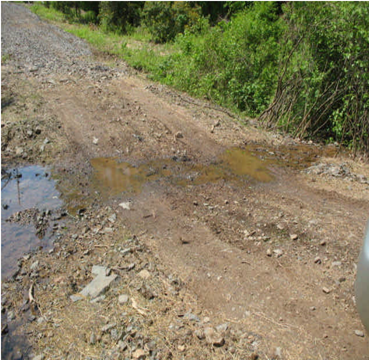
East Mount Rd: Second wetland crossing removed and final graded. Hydrology remains intact but a small amount of sediment was noted downstream.
