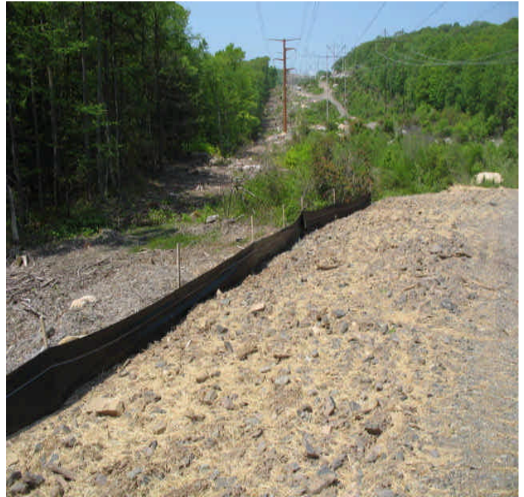
West of Scovill: Final grading and stabilization measures complete. Controls remain in place as needed above sensitive/resource areas. When areas have established cover, silt fence will need to be removed
