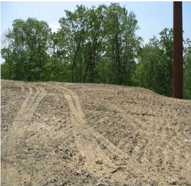
West of Scovill SS: Final grading along the edge of the access road complete.
