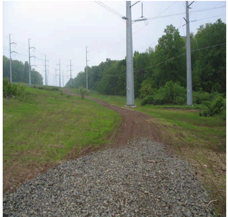
BSS North: Final restoration complete. Grass growth noted in reclaimed areas along the ROW.
