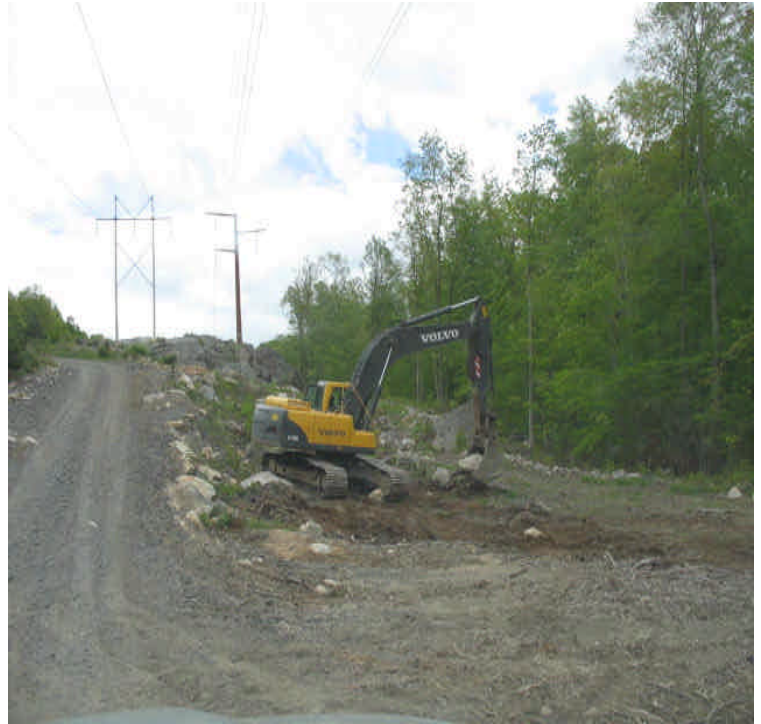
West of Scovill: Final grading and stabilization measures underway. Crews were replacing a section of stonewall.
