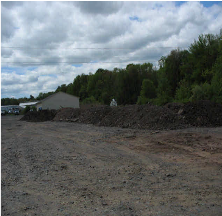
Contractor Yard: Stockpiling soils from restoration at Scovill SS to Chestnut Jct.
