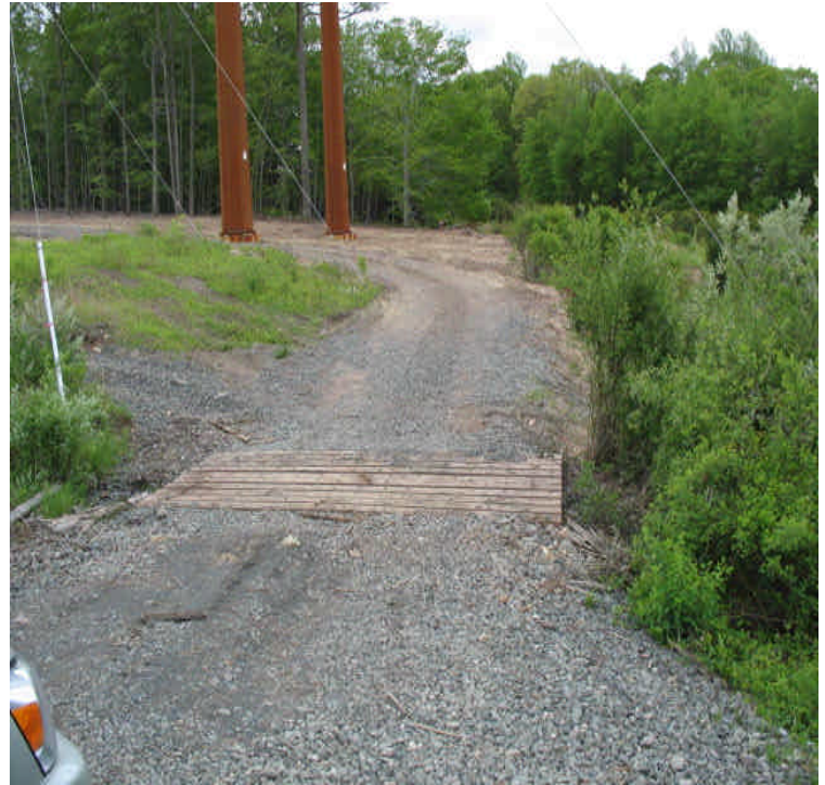
East Mount Rd: Timber mats were replaced in order to access the site and final grading was underway.
