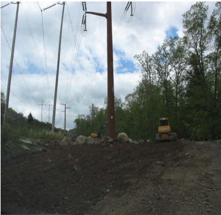
West of Scovill SS: Final grading along the edge of the access road almost complete.
