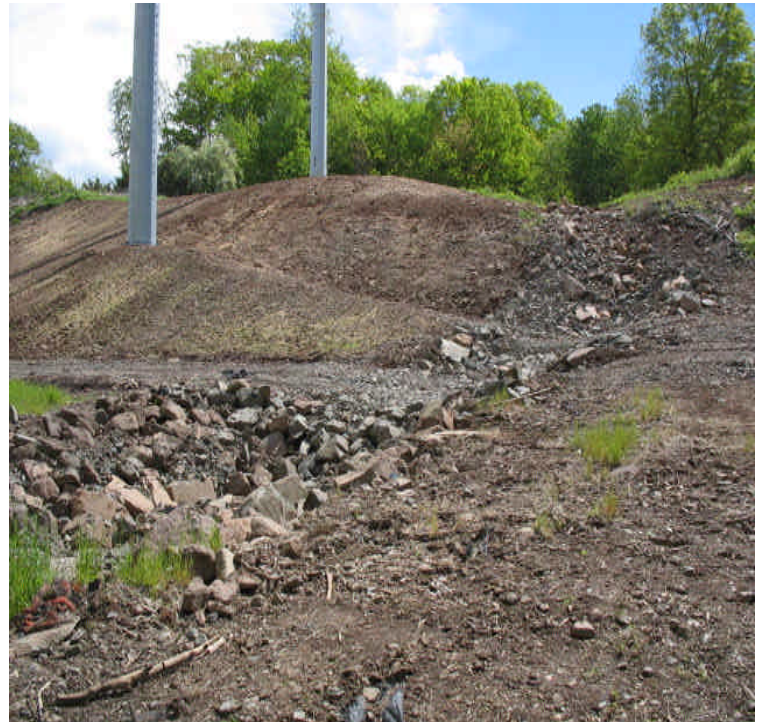
E. Meriden SS (West): Final restoration complete. Riprap settling area and drainage area installed from the runoff near the switching station. Monitor to ensure effectiveness in preventing erosion near the pond.
