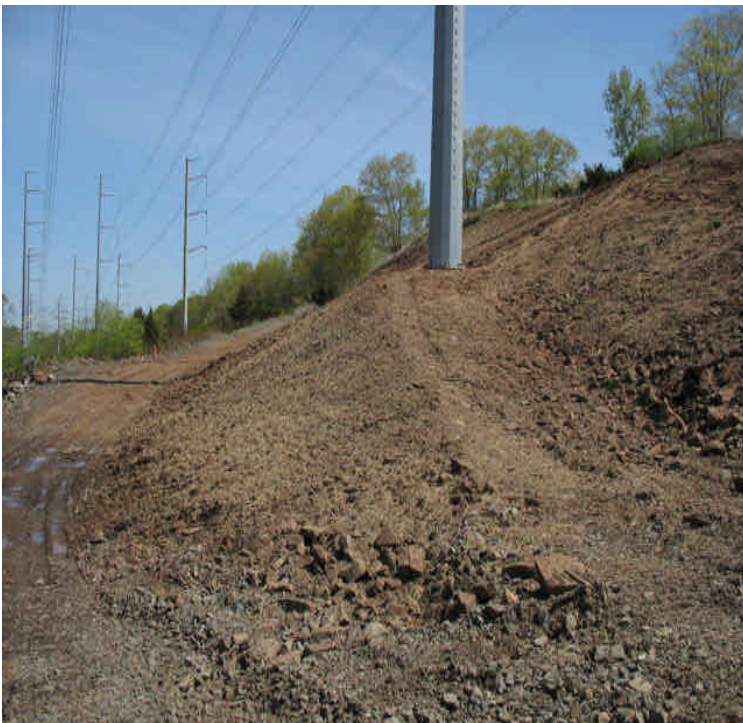
E. Meriden SS (west): Final grading was completed and seed and mulch have been applied at structure #24462. New grading should help minimize erosion issues.
