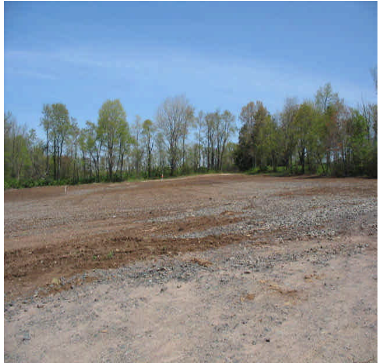
Contractor Yard: Final grading is complete within the field. Measures (mulch/seed) should be applied for stabilization but coordination may be needed with the landowner.
