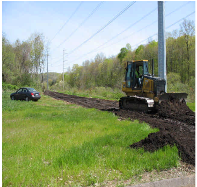
High Hill Rd: Final grading and topsoil application was underway at the western access north of High Hill.
