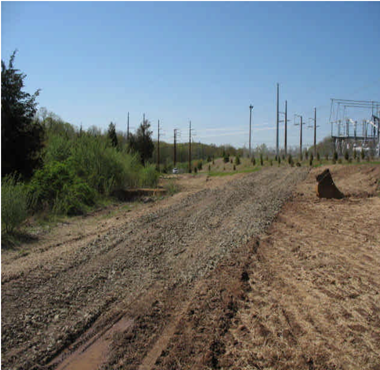
Beseck SS: Old ROW access road has been removed and reclaimed. Access to the ROW was now connected to the BSS eastern access.
