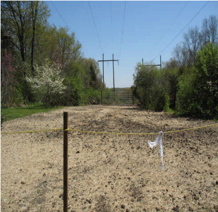
Black Walnut Dr.: Final reclamation is complete at the site entrance. Soils have been seeded and mulched.
