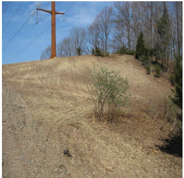
Arbutus St: Restoration and final grading complete west off Arbutus St. Hay/seed have been applied at the last disturbed slope. Add controls along the slope as needed.
