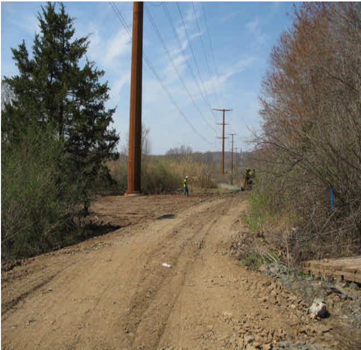
Durham Rd: Timber mats have been removed and contractor is working on the access road.
