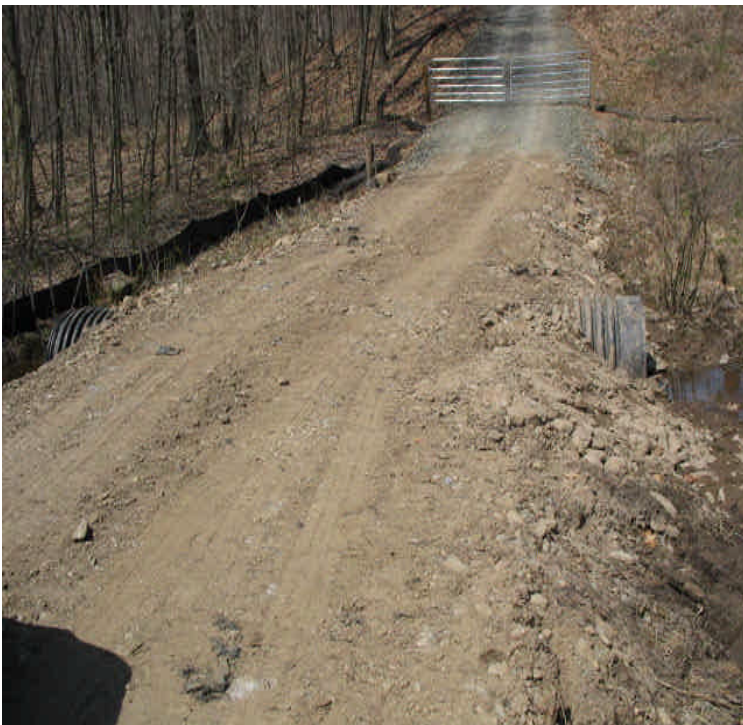
Johnson Ln: A new culvert was installed at the stone wetland crossing to maintain the hydrological connection within the wetland.
