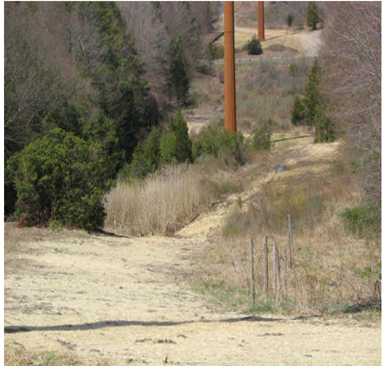
Foot Hills Rd: Timber mats and access road were removed within the ROW and wetlands and the areas were reclaimed. Mulch and seed were applied.
