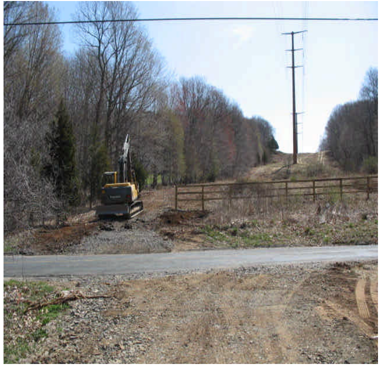
Arbutus East: Final grading and access road work is underway. Stabilize the exposed areas as needed and continue to monitor.
