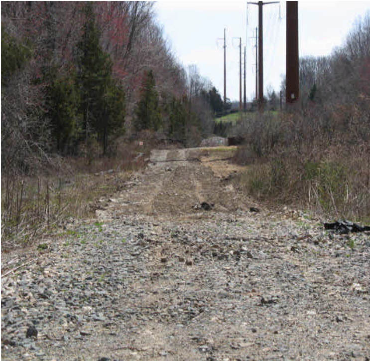
Haddam Quarter Rd: Timber mats were removed from the wetland crossing. Stone and soil were installed for the permanent access road. Consider installing culverts in this area to avoid altering wetland hydrology.
