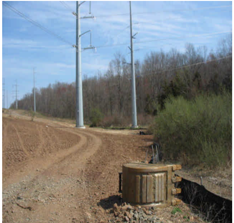
Beseck SS North: Final restoration and access road removal complete from BSS north. Monitor for final stabilization through vegetative cover Access road and final restoration still needed east of BSS.
