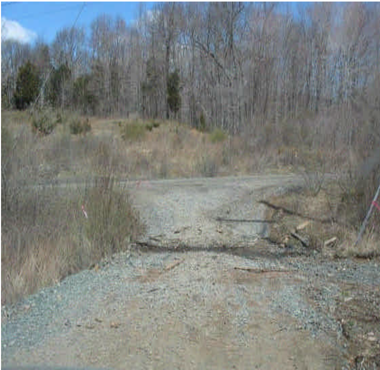
E. Mount Rd: Timber mats were removed from the wetland crossing at the E. Mount entrance. However, future access still appears to be needed and the crossing will need to be replaced.
