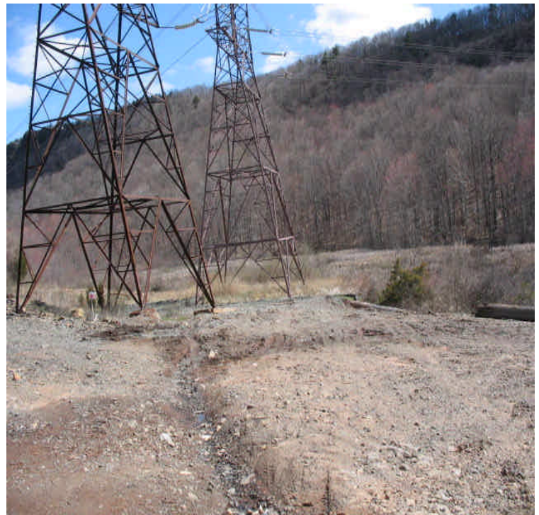
Black Pond Jct: Drainage channels and repaired controls appear to be working well. Stabilize/reclaim this area as soon as possible.
