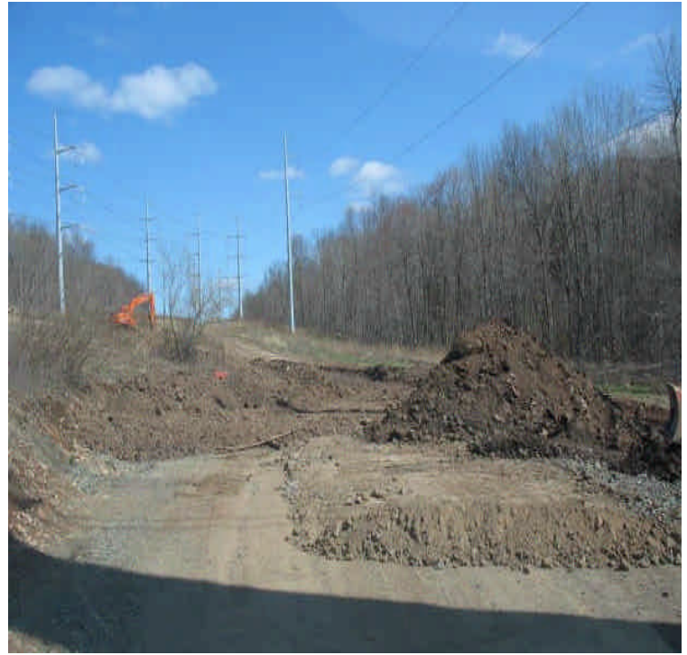
North of Beseck SS: Final grading and access road work is underway. Stabilize exposed areas as needed and monitor the area.
