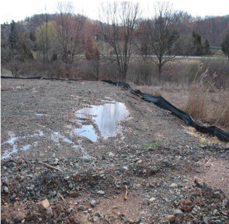
North of E. Main St: Controls are still in place along the wetlands and The new drainage channel is working well. These areas are waiting for reclamation.
