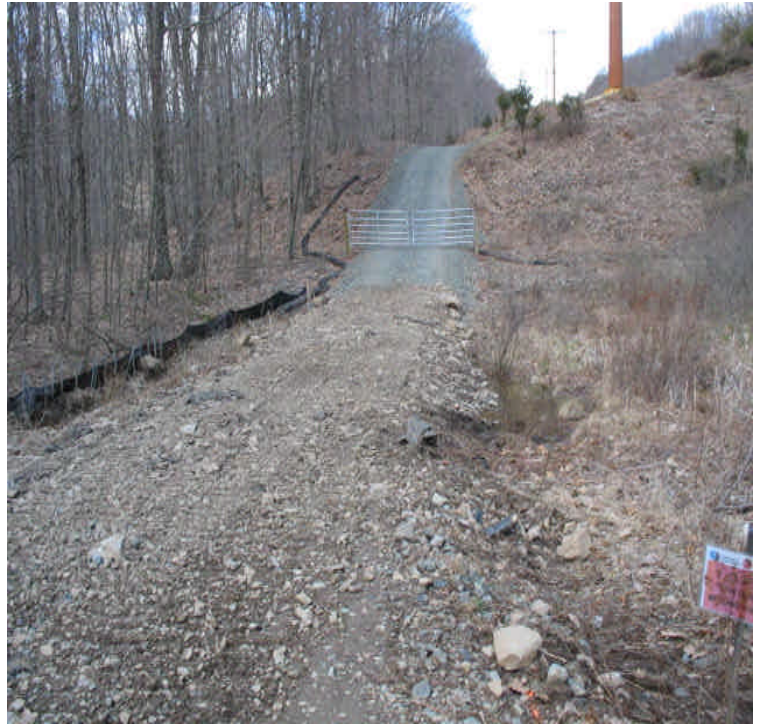
Johnson Ln: Timber mats and culvert were removed from the wetland crossing. A new permanent stone access road was installed, effectively bisecting the wetland and blocking hydrology. A culvert should be added.
