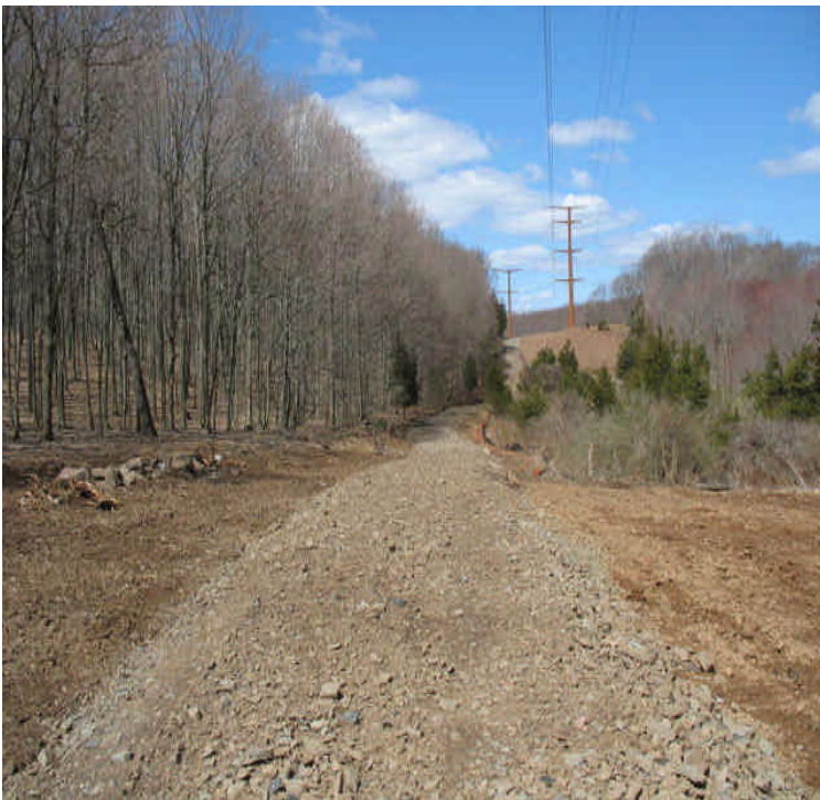
Arbutus St: Timber mats were removed and a new permitted stone access road was installed at the edge of the wetlands. Stabilize exposed soil as needed.
