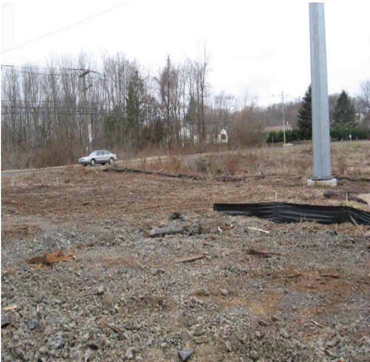
North of High Hill Rd: Reclamation and final grading is still needed in some areas. Final restoration will continue from BSS north.
