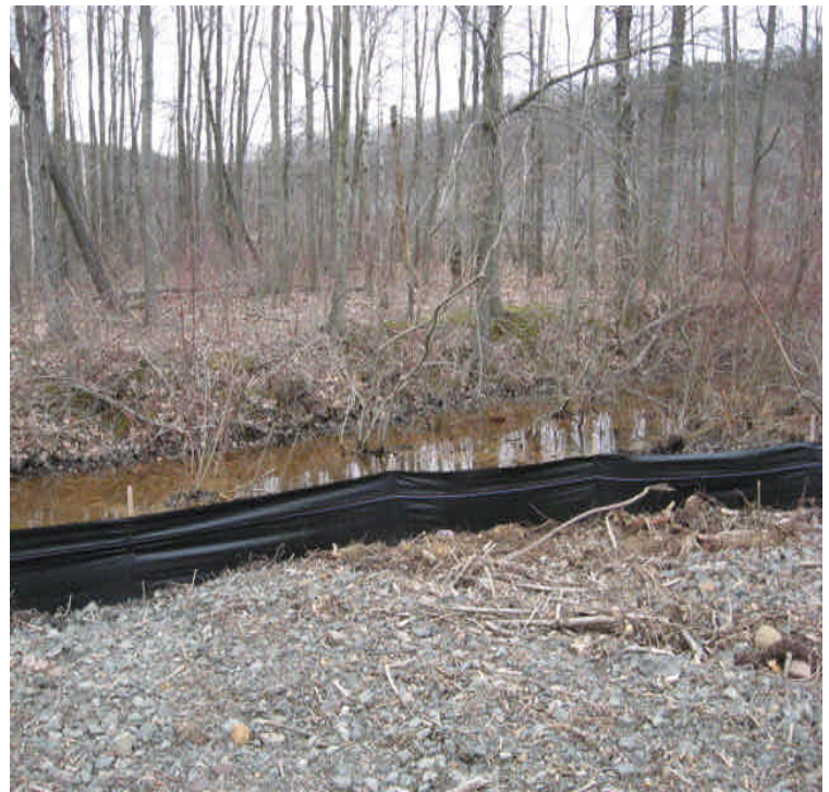
South of E. Main St: Adjacent stream is clear and controls remain in place at a pad waiting for reclamation.
