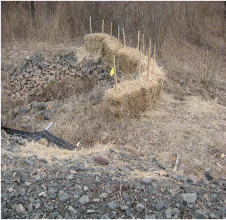
East of BSS: Controls at the outlet appear to be holding up. No turbid water has been observed leaving the basin since the controls were installed. (However, recent rain events have not been significant).
