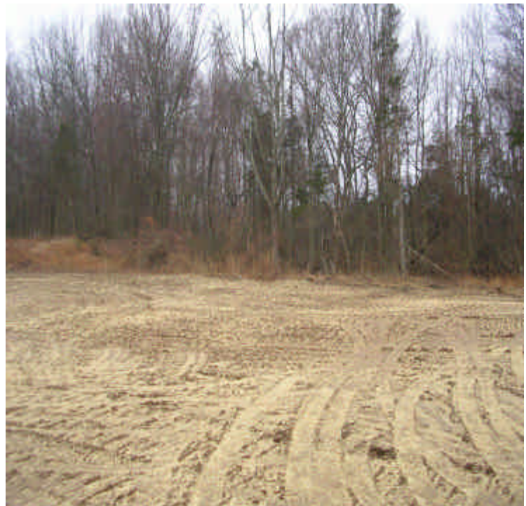
Black Walnut Dr: Several exposed areas continue to be graded, mulched and seeded.
