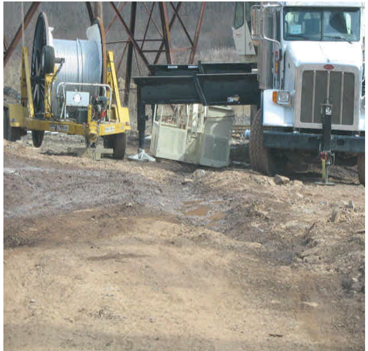
Black Pond Jct: Turbid water from the access roads and slopes are being redirected away from wetlands. Controls along the wetlands have been repaired/reinforced as needed.
