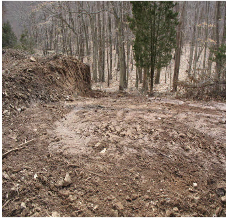
Black Walnut Dr.: Exposed slope from recent reclamation and grading. Crews were reducing the overall grade of the slope during this process. Water bars were installed to divert flow in this area. Additional stabilization is needed upon completion of work.
