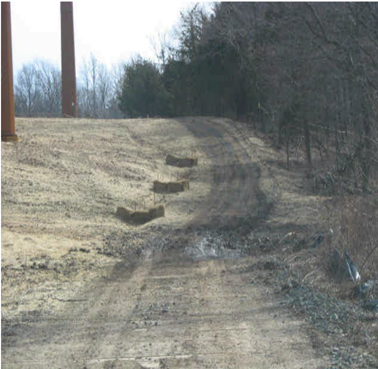
Powder Hill Rd: Reclamation and final grading is complete in some areas. Haybale check dams were added to a drainage ditch to filter and control stormwater.
