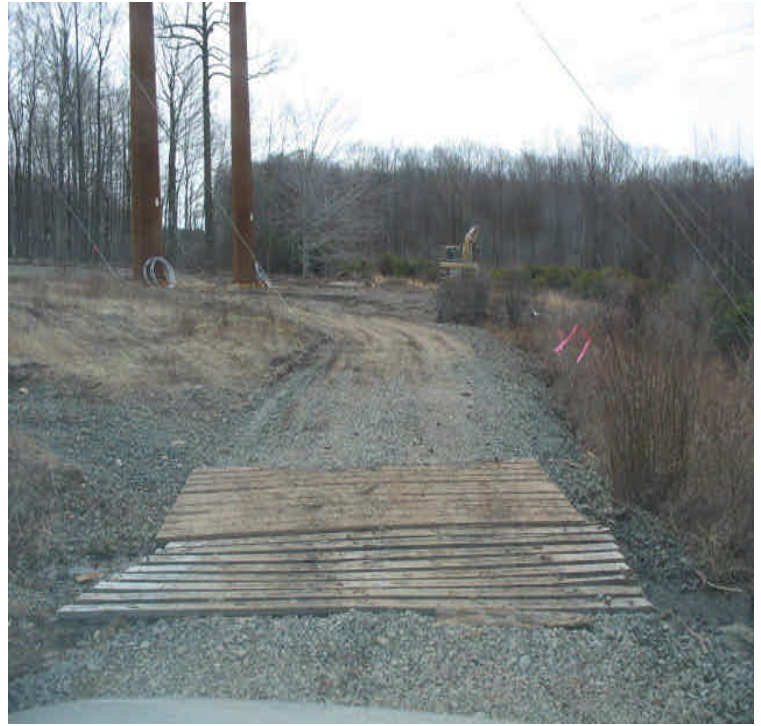
East Mount Rd: Stone and timber mats were added to the access road entrance at the saturated crossing
