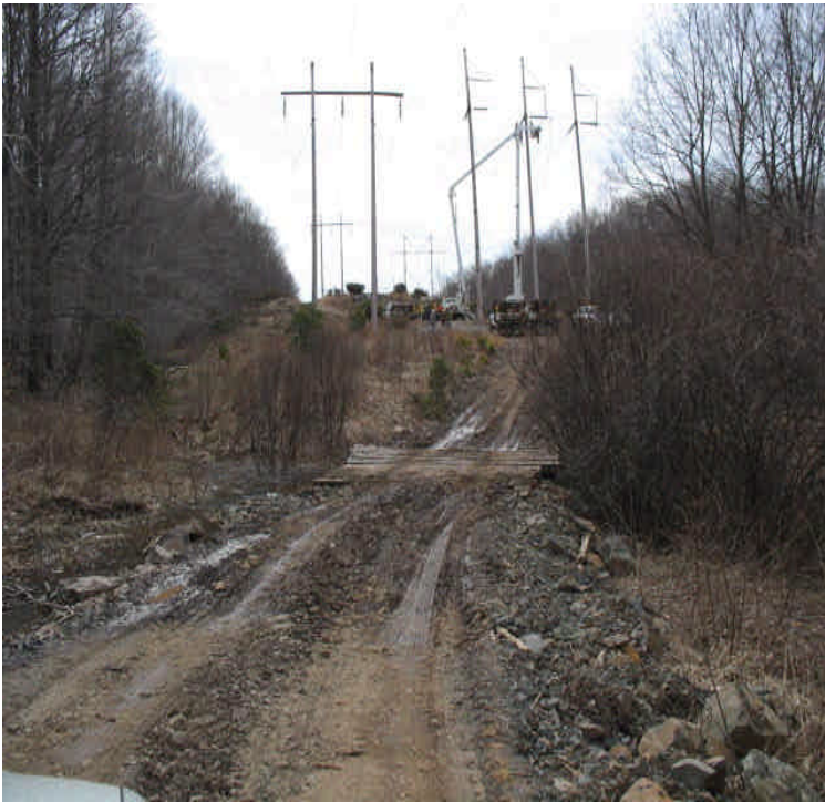
East Mount Rd: The new section of access road noted south of East Mount Rd. extends through a saturated crossing. Timber mats were installed to allow water to flow in its original path across the access.
