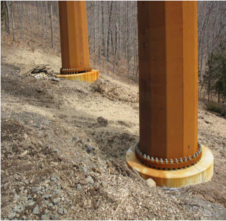
Black Walnut Dr: Reclaiming and regrading were occurring along the slope. Exposed soils were mulched and seeded. Continue to monitor since the slope has high erosion potential.
