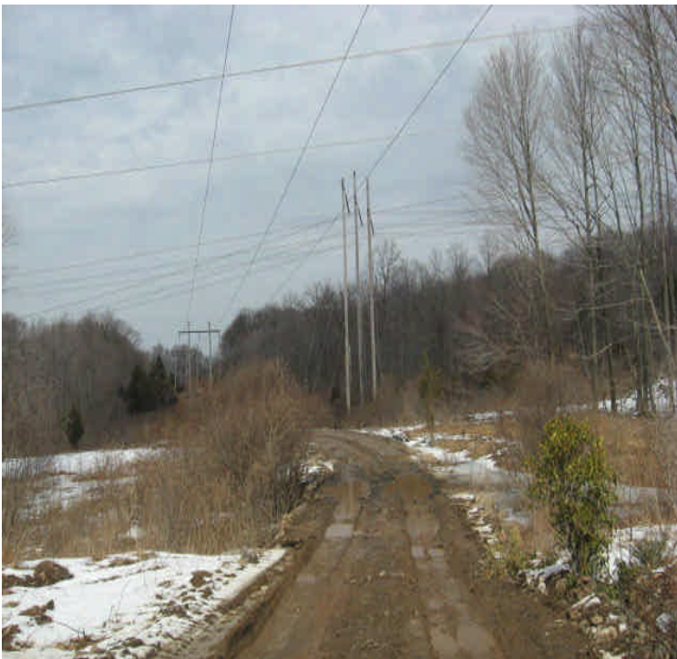
East Mount Rd: New section of access road extending through a saturated crossing, with water becoming turbid and flowing off site.
