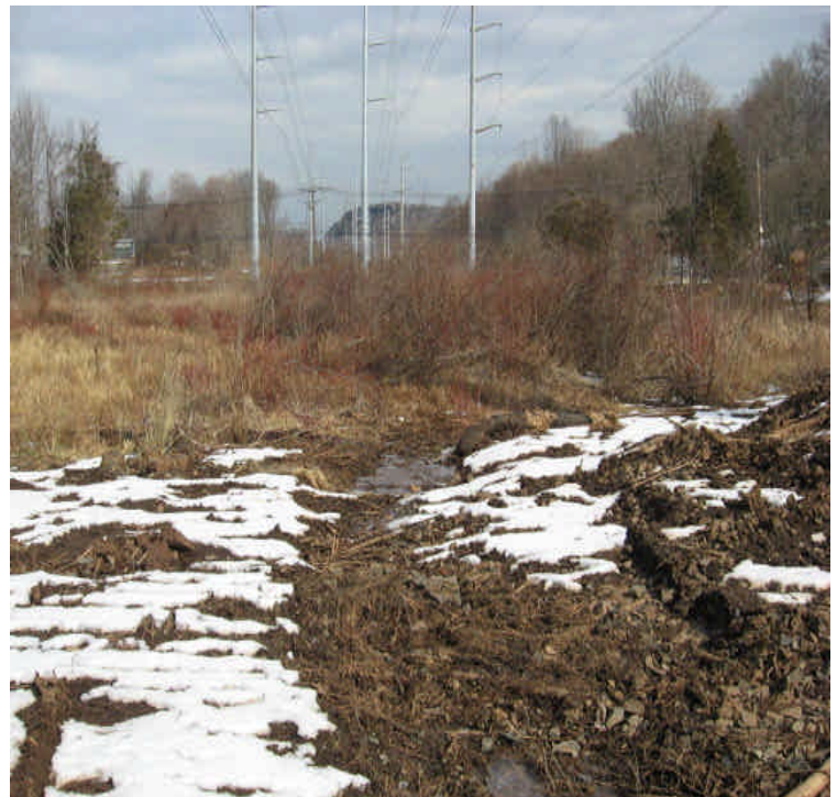
South of High Hill: Timber mats were removed from the wetland. A few gaps in controls were noted and should be repaired at this time. Crews are planning full restoration of areas in a linear fashion in this section.
