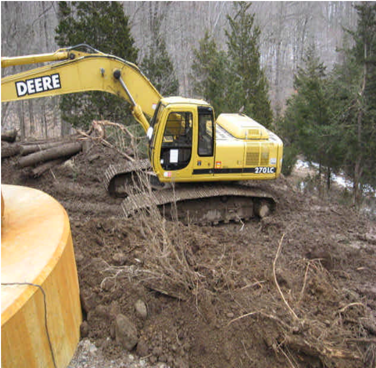
Black Walnut Drive: Additional grading upgradient from Ball Brook. The area currently needs more controls and the soils and erosion-prone slope will need careful stabilization when work is complete.
