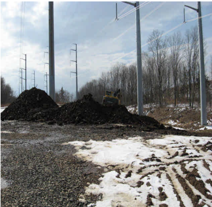
North of E. Meriden SS: Crews were reclaiming pad sites and removing mats and stone from above the second stream channel.
