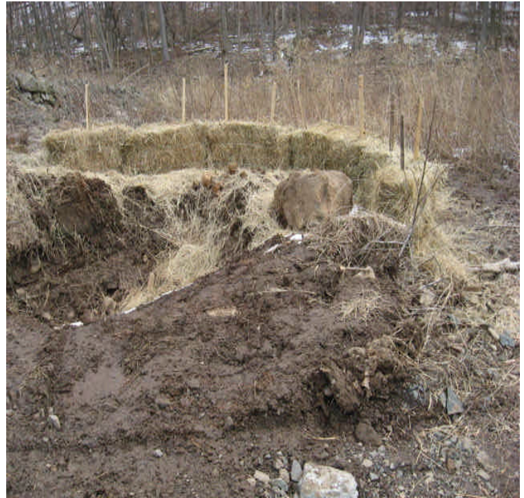
North of Beseck SS: Drainage ditches/water bars and settling basins have been regraded. New haybales were also installed.
