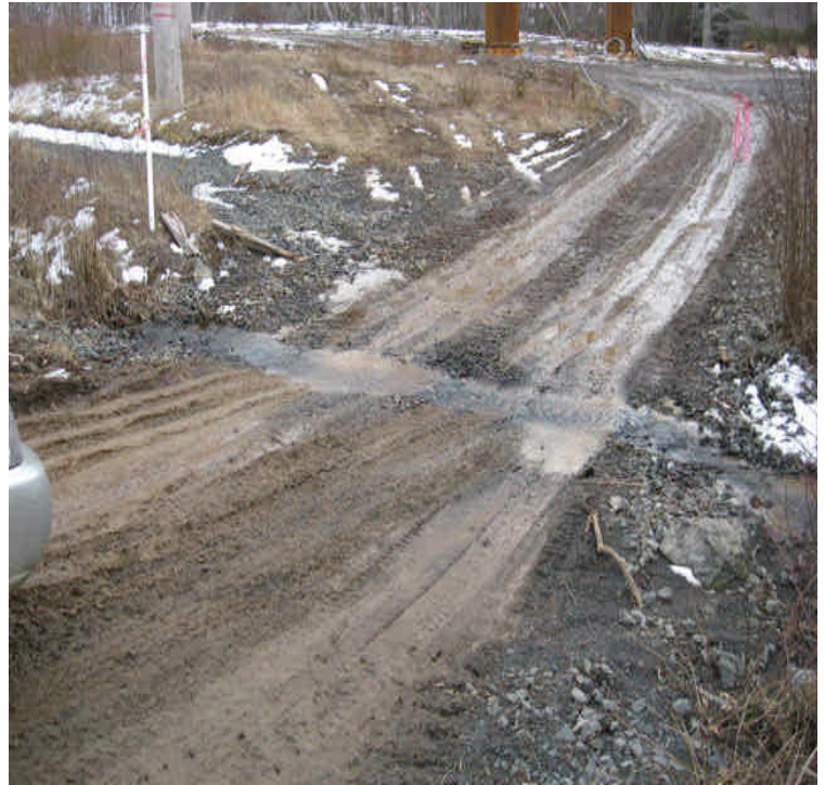
East Mount Rd: Run-off continues to flow at the saturated crossing, becoming slightly turbid across the access road.
