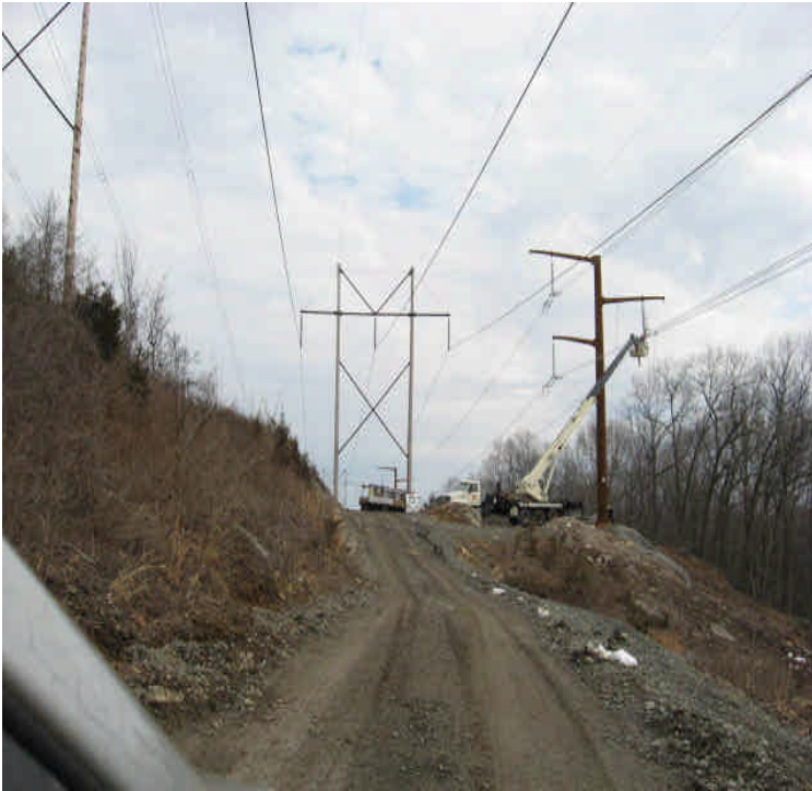
West of Scovill SS: Wetland #5 crossing is in good shape. Line work was underway.
