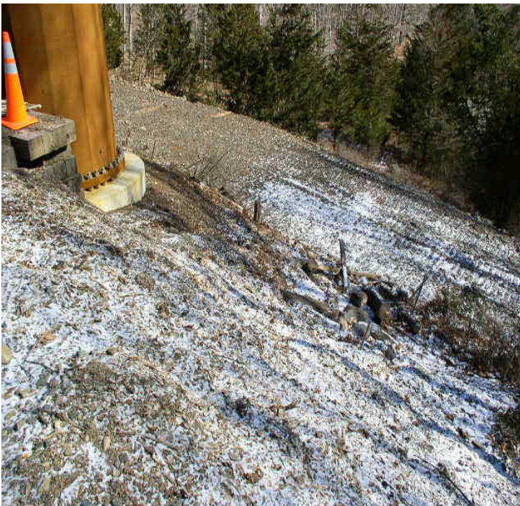
Black Walnut Dr: Grading noted around the last structure before Ball Brook to accommodate line pulling equipment.
