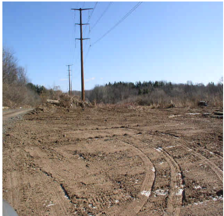
Little Ln: Wooden structures removed, final grading is complete. Temporary stabilization measures needed on exposed soils.
