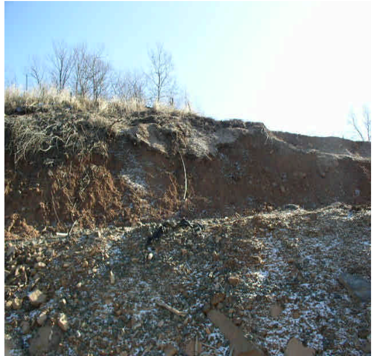
East Meriden SS: Erosion noted on the steep slopes at structure 2446. Run-off remains contained to the ROW but stabilize when feasible.
