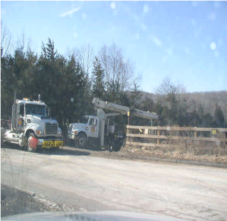
Powder Hill Rd: Sediment tracking was noted on the roadway. Equipment removal from this section was underway.
