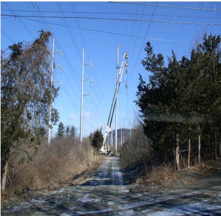
North of High Hill: Insulator installation continues moving toward Black Pond Jct.
