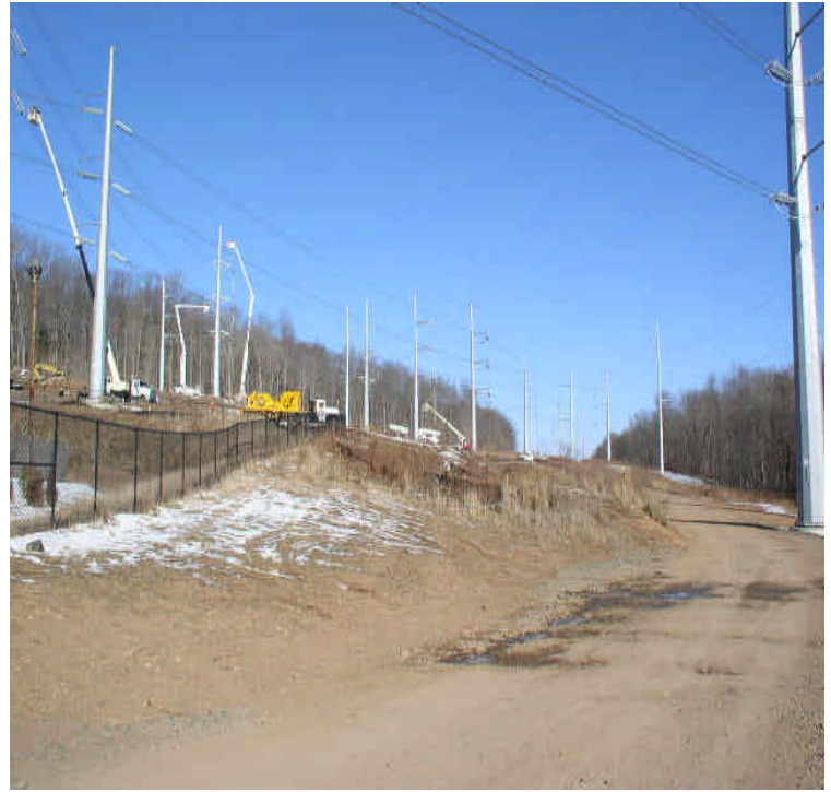
North of Beseck SS: Line work underway moving north from the switching station.
