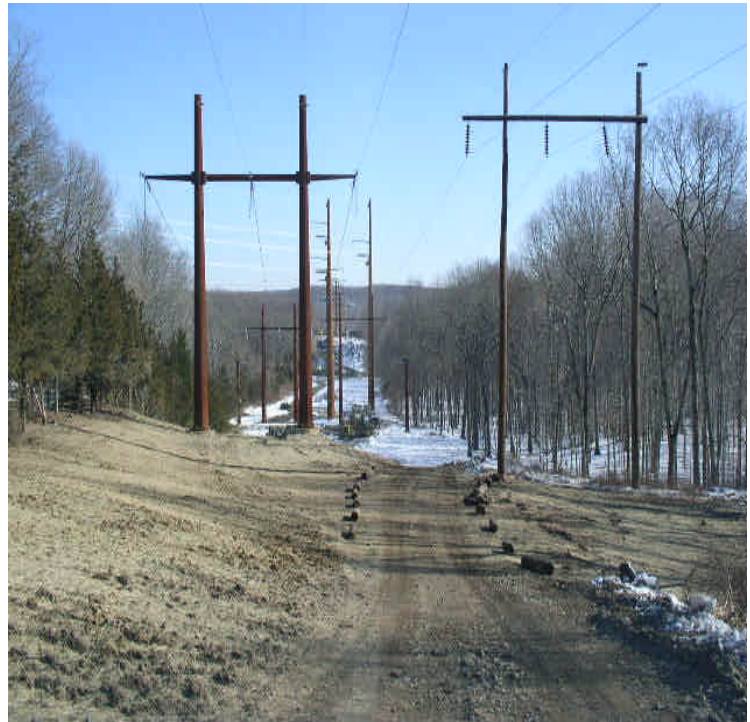
Black Walnut Dr: Final grading completed adjacent to the access road. Hay mulch and seed have been applied in reclaimed areas.
