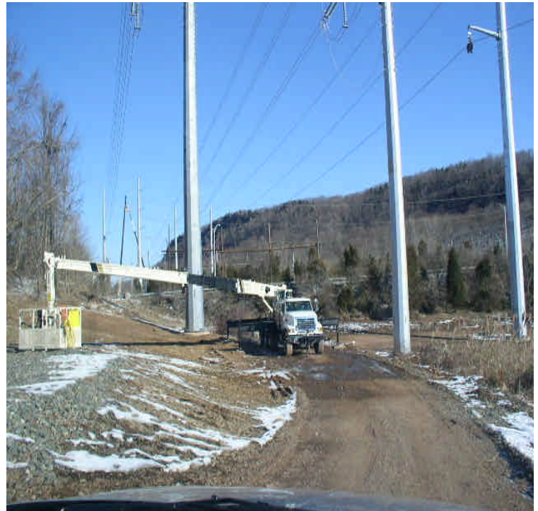
North of East Main Street: Line workers were preparing to install insulators.
