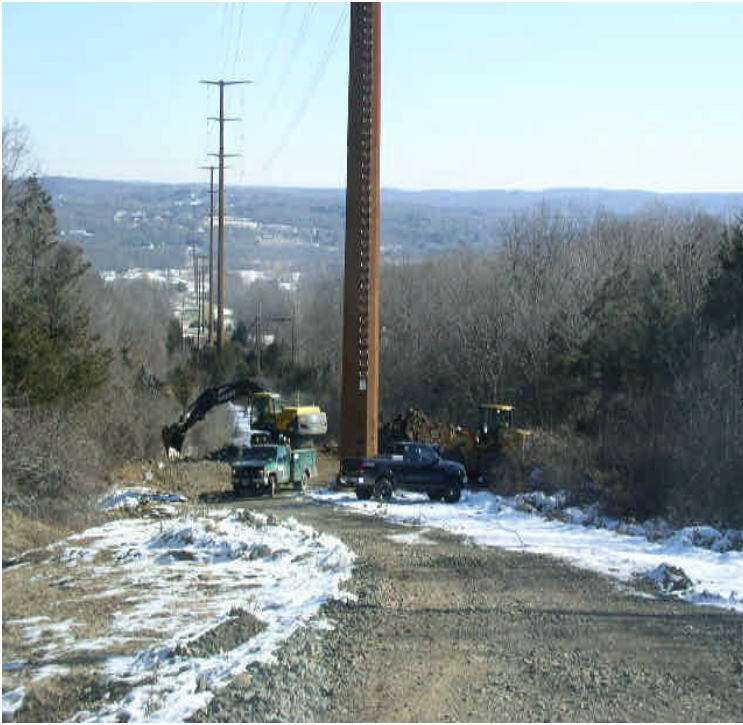
Powder Hill Rd: Minor pad work and restoration work underway east of the roadway.
