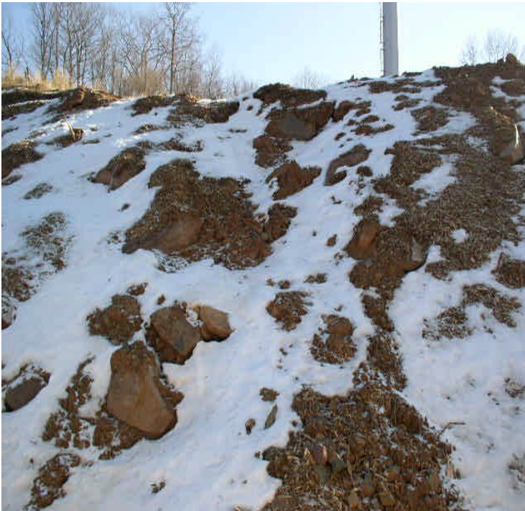
E. Meriden SS: Line work was underway. Small eroded, rill channels were forming along a pad slope. Run-off was contained to site but provide stabilization when conditions permit.
