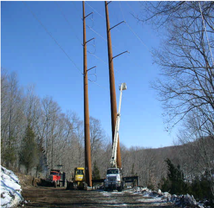
Black Walnut Dr: Minor pad work underway in preparation for line pulling activities.
