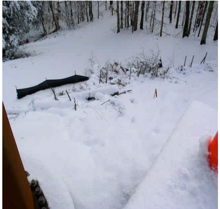
Controls remain upgradient from Ball Brook at the end of the Black Walnut Dr. entrance access road.
