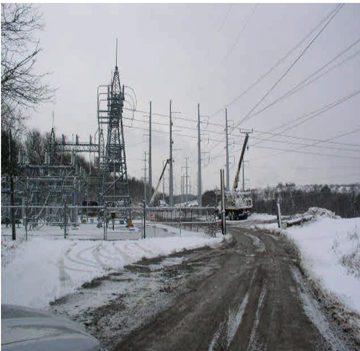
E. Meriden SS: Line work underway between here and Black Pond Jct.
