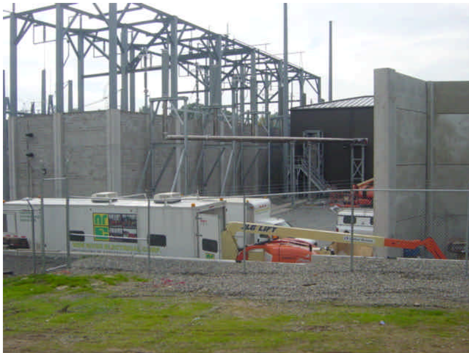
Tie-in work continues inside the Norwalk substation. New River Electric was on-site performing work.
