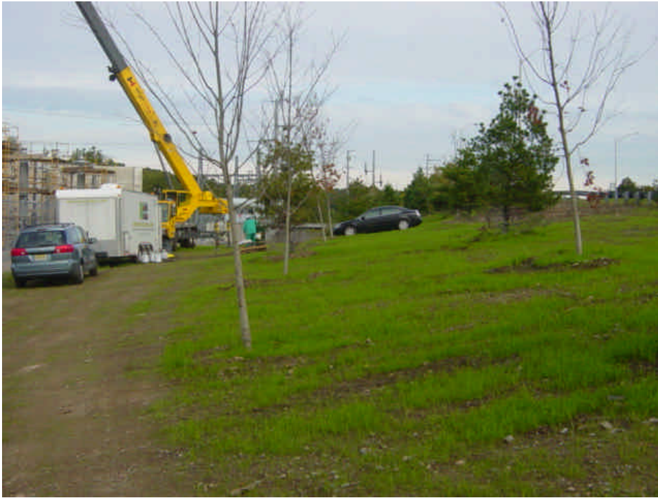
Crane was onsite to set electrical equipment at the Norwalk Substation. New River Electric was also on-site.
