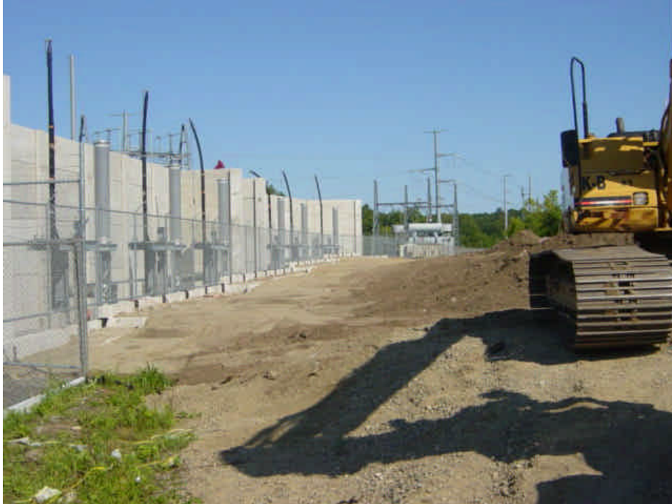
Electrical tie-in work continues inside the substation. Pre-cast concrete retaining wall has been reset along the substation perimeter.
