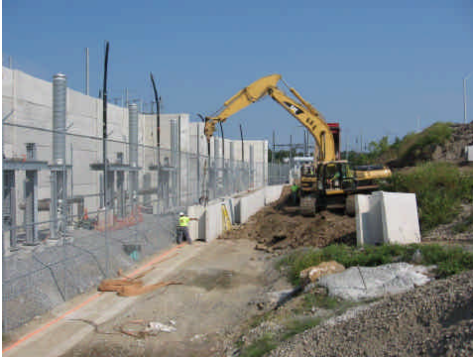
Electrical tie-in work continues inside the substation. Pre-cast concrete retaining wall was being reset on the outside of the substation.
