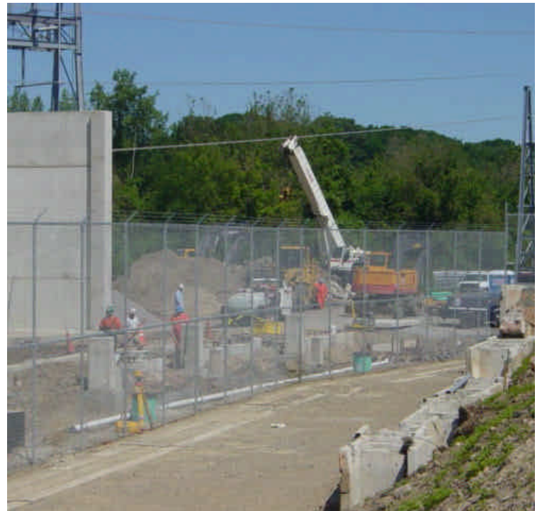
Stockpiles remain adjacent to the work area but there were no observed erosion issues. Watch any adjacent catch basins within the yard as they outlet to the river.
