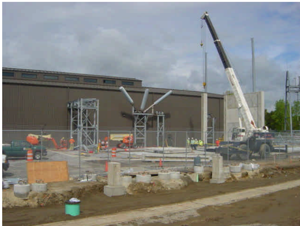
A steel structure was being installed next to the existing GIS building at the time of the inspection.
