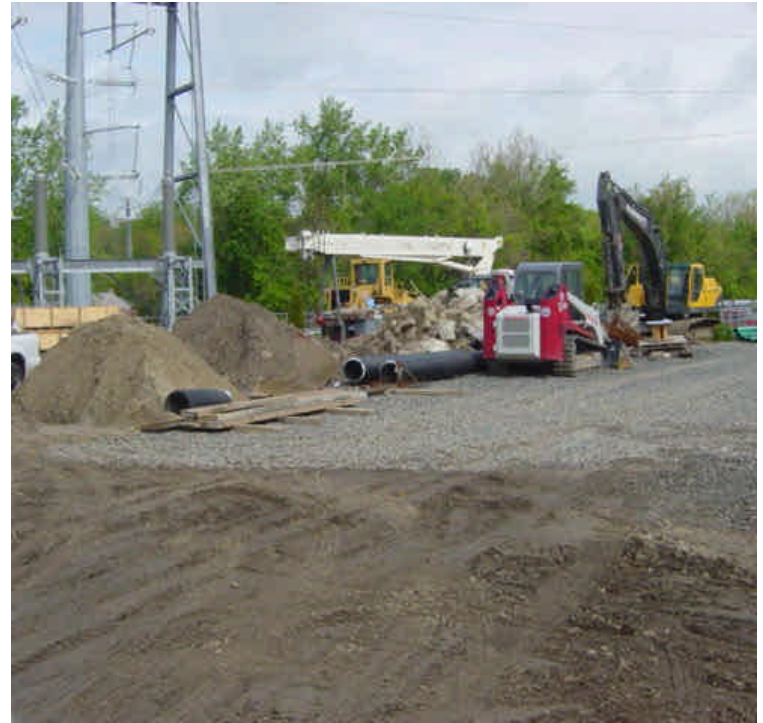
Several stockpiles of material were observed without appropriate containment immediately at their base, but they do remain contained to the yard.
