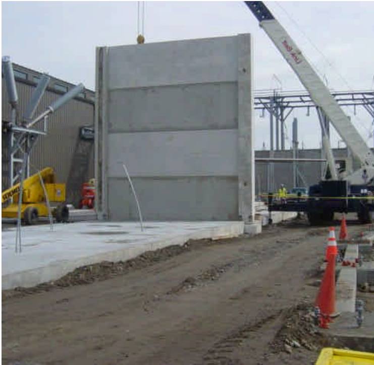
Crews were setting pre-cast concrete wall segments on the previously placed foundation slab.
