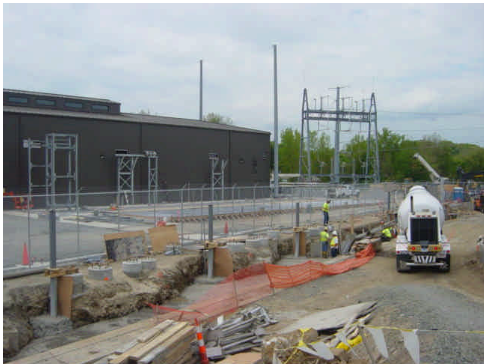
The concrete slab that was being formed during last week's inspection has been poured.
