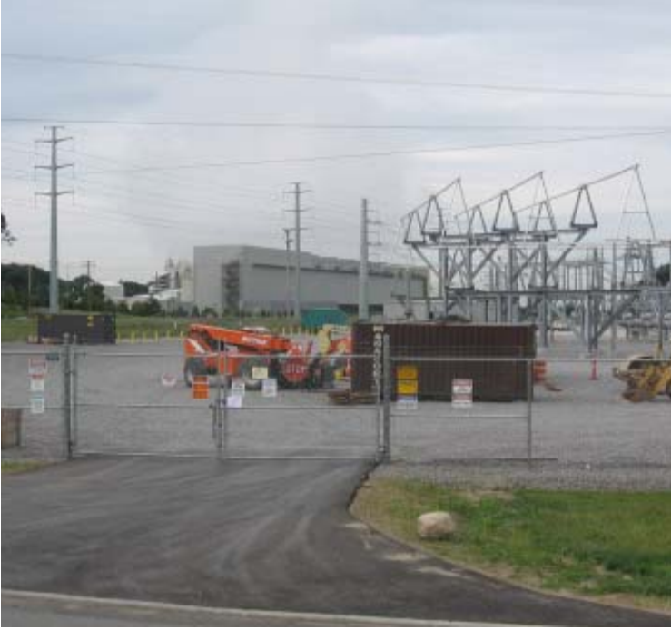
East Devon Substation (Milford): A view of the northern portion of the substation. Both northern access points have been paved with asphalt.
