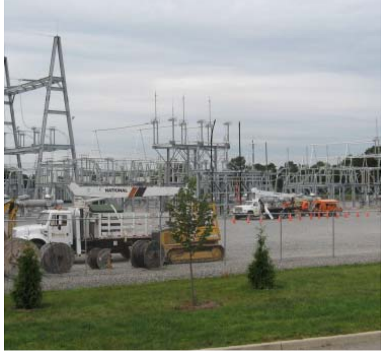
East Devon Substation: A view of the vegetative growth along Plains Rd and a general view of construction at the substation.
