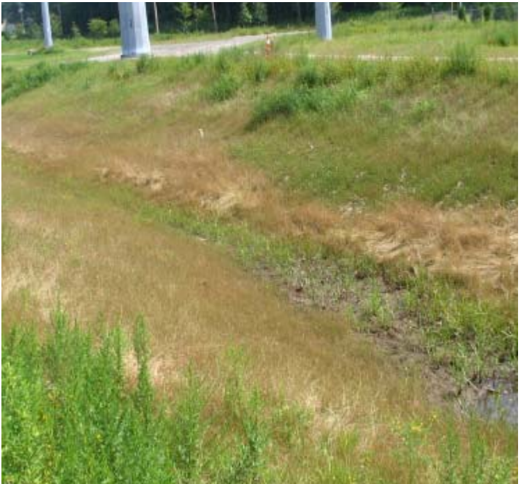
East Devon Substation: The vegetated swale remains stable.
