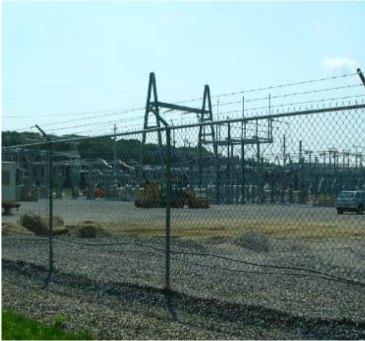
East Devon Substation (Milford): A view of the northern portion of the substation. Construction continues here.
