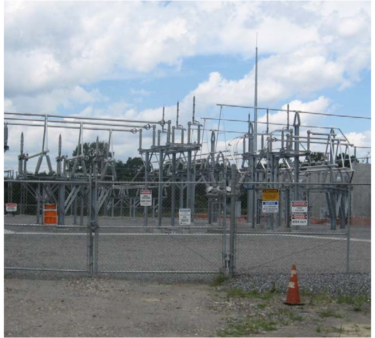
East Devon Substation: An additional view of the southern portion of the substation.
