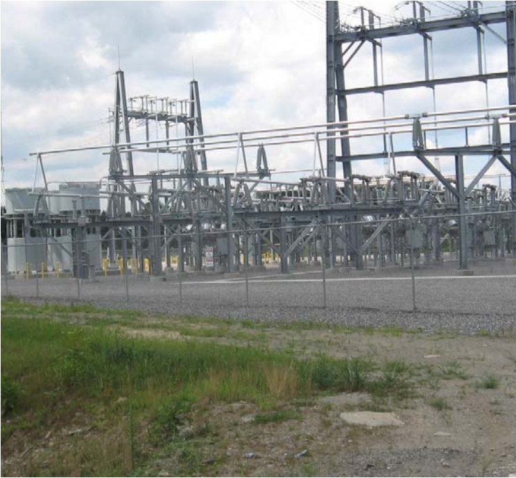
East Devon Substation (Milford): A view of the southern portion of the substation. Construction is complete in this section.
