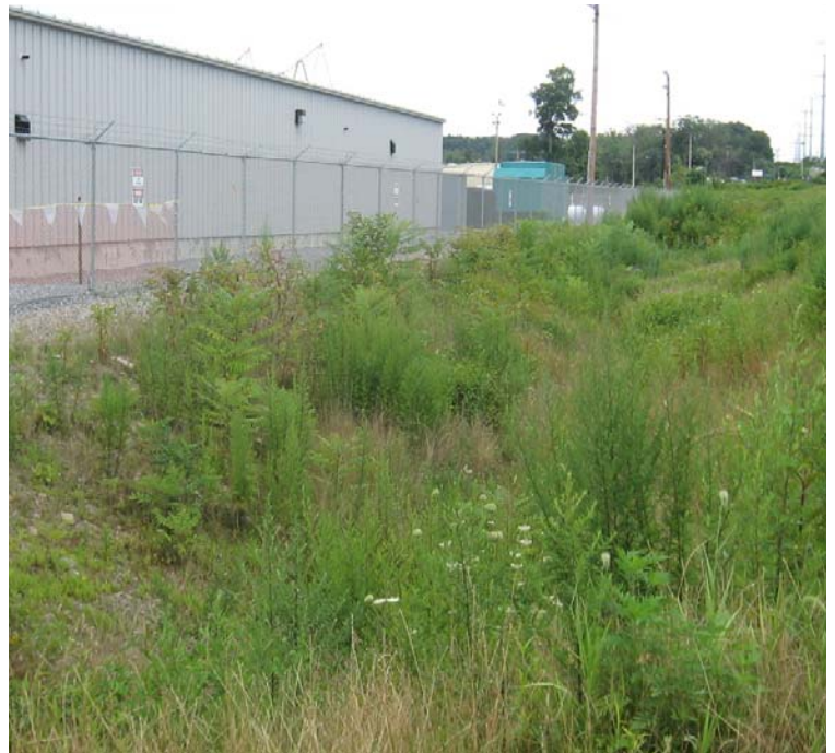
East Devon Substation: The central portion of the vegetated swale is stabilized with approximately 90% vegetative cover.
