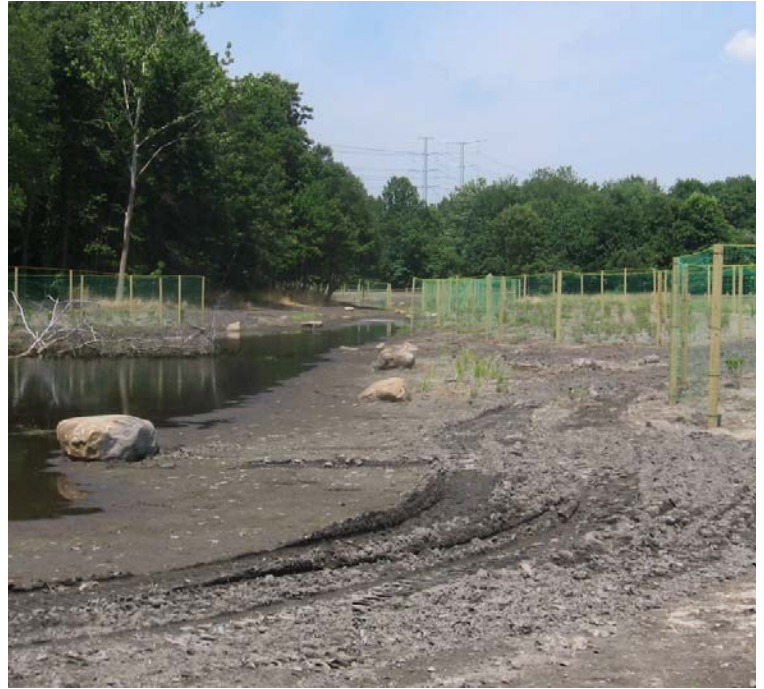
Wetland Mitigation Area: A general view of the eastern side of the mitigation area. Deer fence installation is complete.
