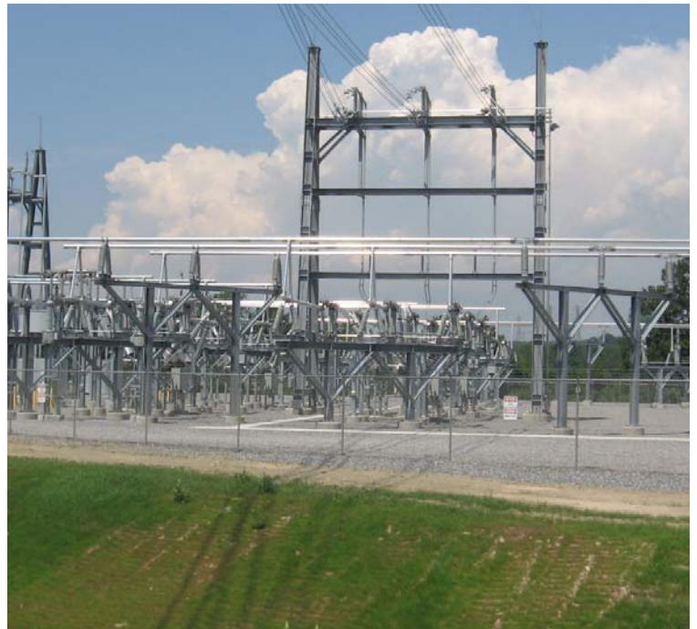
East Devon Substation: A view of the southern portion of the substation site.
