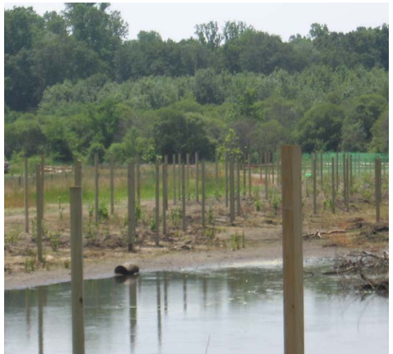
Wetland Mitigation Area: An additional view of the plantings and deer fence installation.
