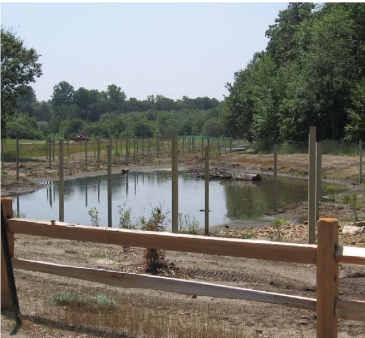
Wetland Mitigation Area: A view of the plantings and deer fencing installation.
