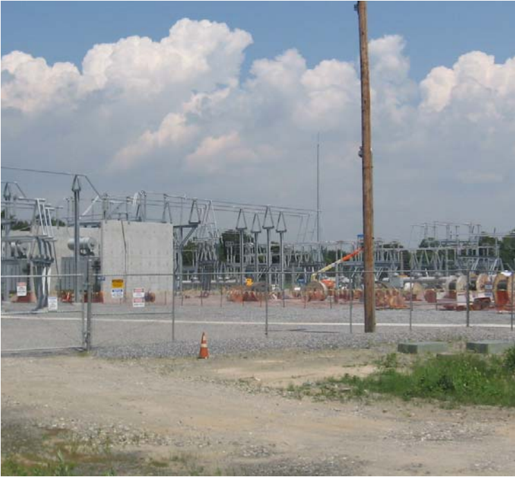
East Devon Substation: A view of the northern portion of the substation site.
