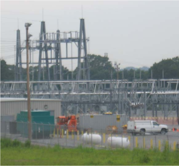
East Devon Substation (Milford): A general view of construction at the substation site.
