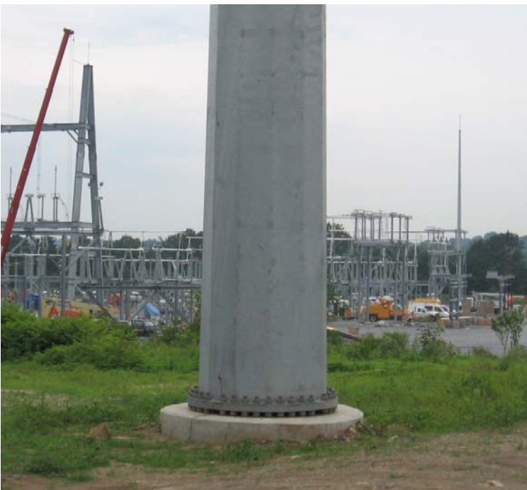
East Devon Substation: A view of the substation looking south from Plains Road.
