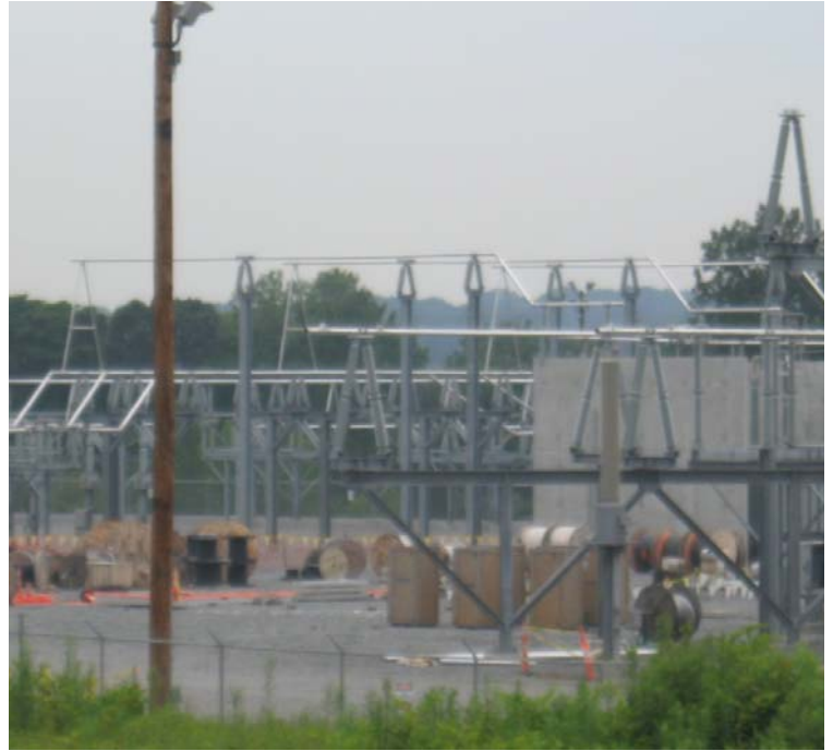
East Devon Substation: An additional view of construction at the substation site.
