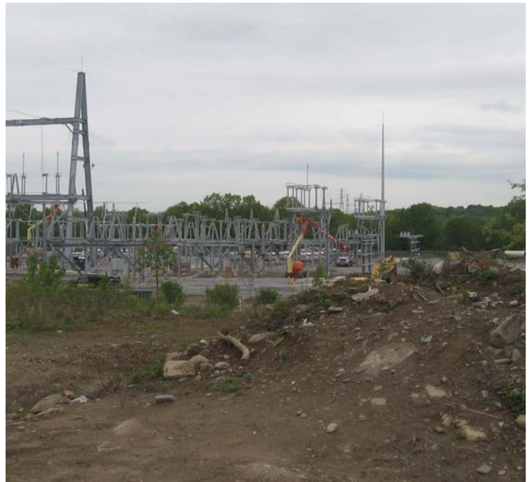
East Devon Substation: A view of construction at the substation from Plains Rd.
