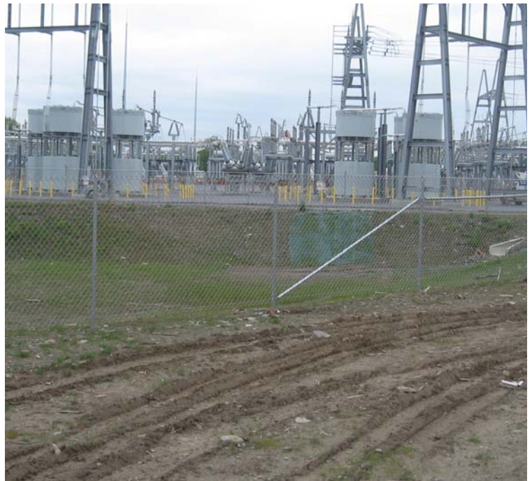
East Devon Substation: An additional view of the detention basin and construction at the substation.
