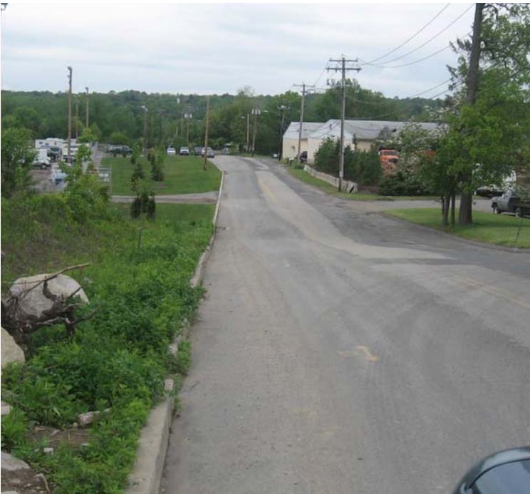
East Devon Substation: A view of Plains Rd. No tracking from the site was observed this week.
