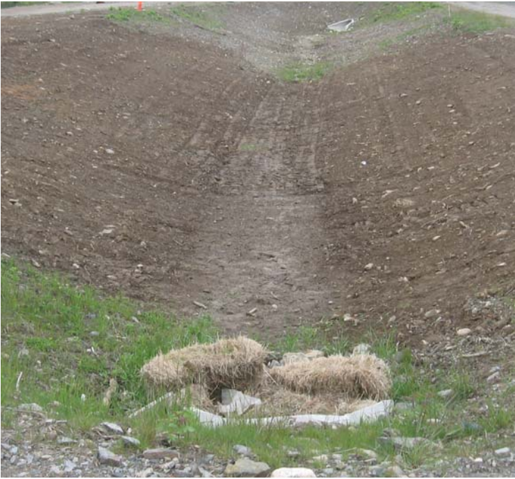
East Devon Substation: A view of the southern portion of the vegetated swale. Exposed soils remain from construction.
