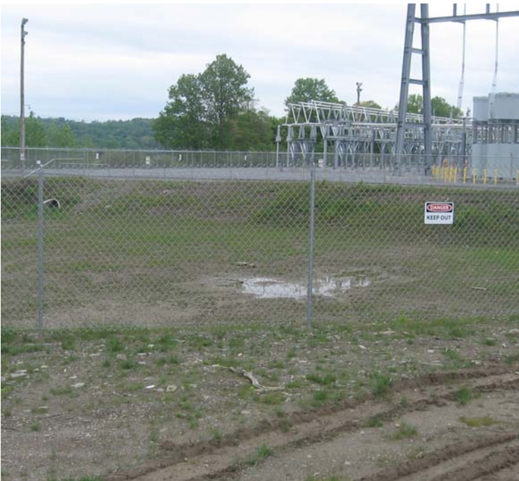
East Devon Substation: A general view of the detention basin and construction at the substation.
