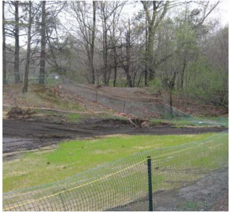
Eisenhower Park: Construction of outflow structures from the mitigation site to the Wepawaug River was active this week.
