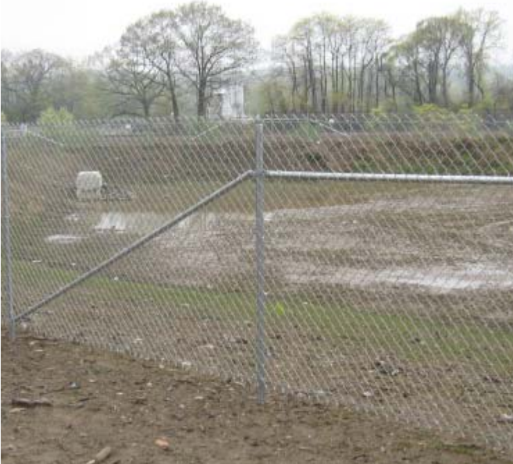
East Devon Substation (Milford): A view of the detention basin located along the southern boundary of the substation.
