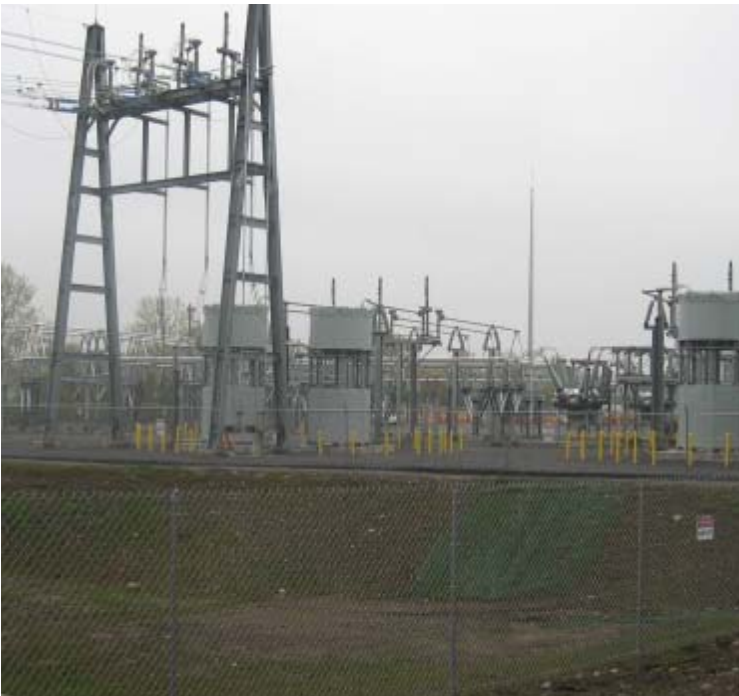
East Devon Substation: A general view of construction at the substation site.
