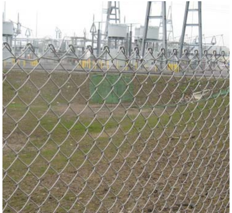
East Devon Substation: Some vegetative growth has been noted within the basin.
