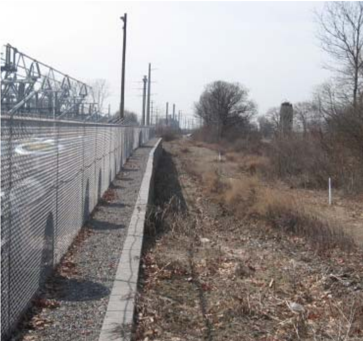
East Devon Substation (Milford): A view of the retaining wall located along the western boundary of the substation.
