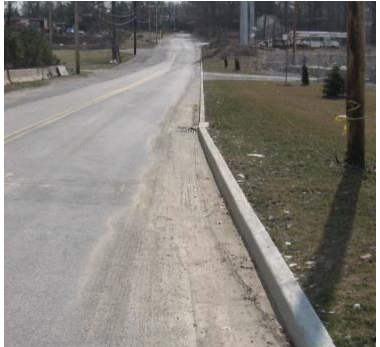
East Devon Substation (Plains Rd): Sediment from the substation is accumulating in the roadway and around the catch basins.
