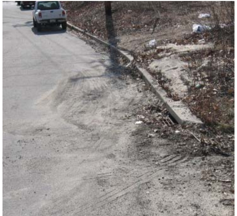
East Devon Substation (Plains Rd): Sediment is accumulating near the catch basin located at the end of Plains Rd.
