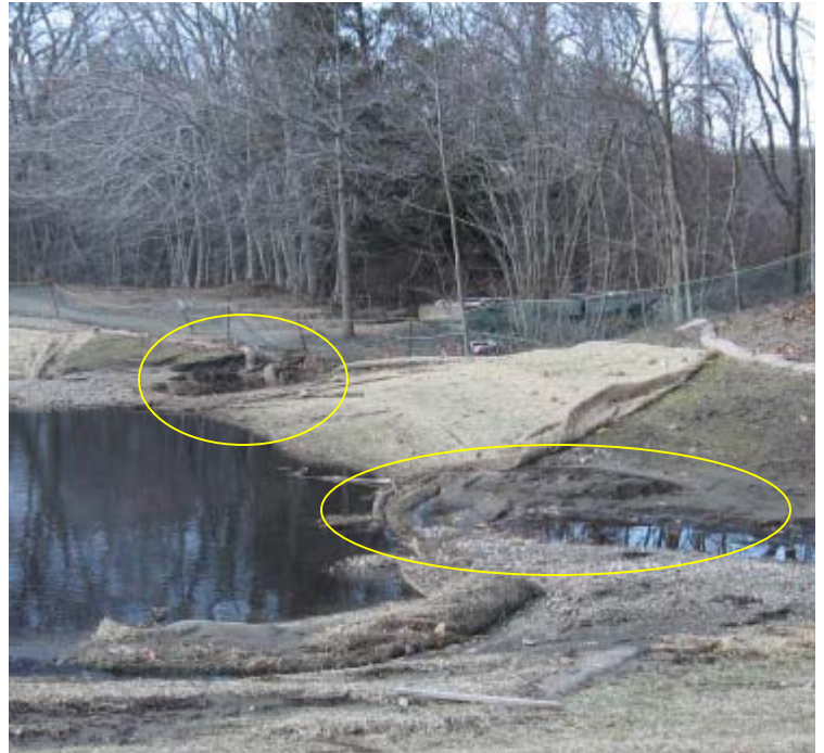
Eisenhower Park: Floodwaters from the Wepawaug River have created two erosive gullies along the bank of the mitigation site.
