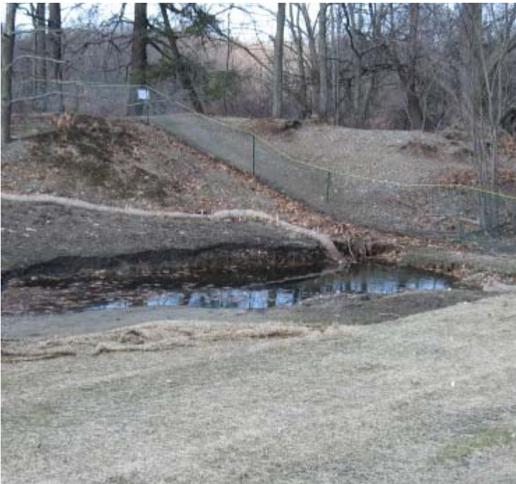
Eisenhower Park: A view of the erosive gully located just west of the access road.
