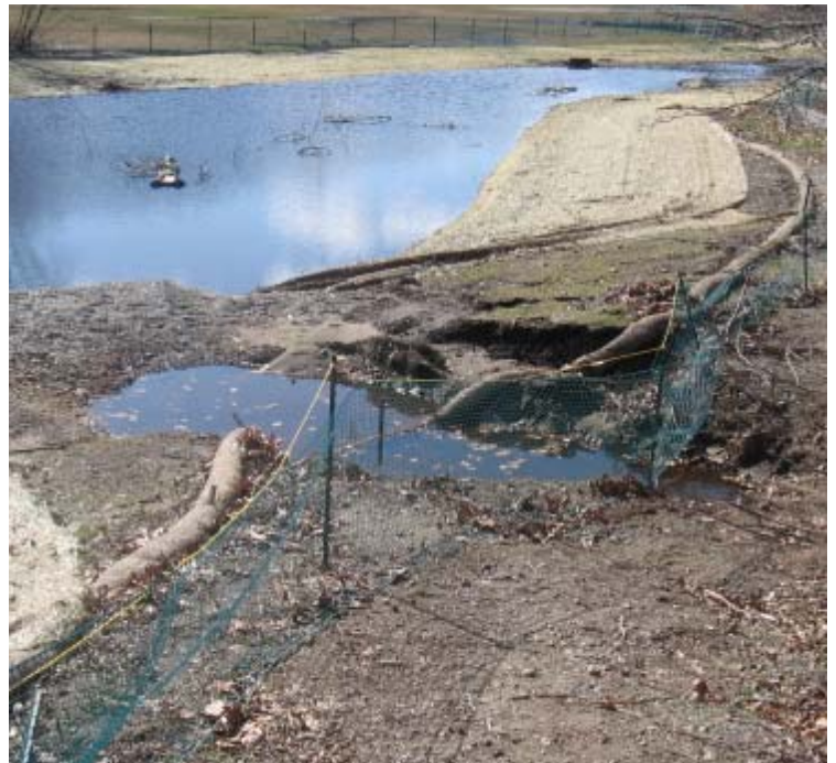
Eisenhower Park: This gully is located approximately 100 feet west of the access road. At this time, it does not appear that sediment has migrated from the mitigation site to the Wepawaug River.
