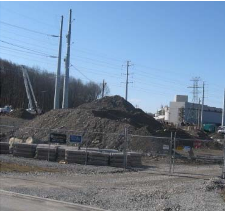
East Devon Substation: The spoil pile remains in the northeast corner of the substation site.
