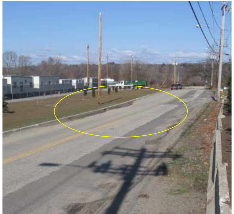
Plains Rd (Milford): Sediment tracking from the substation was evident this week. Sediment is accumulating around the catch basins.
