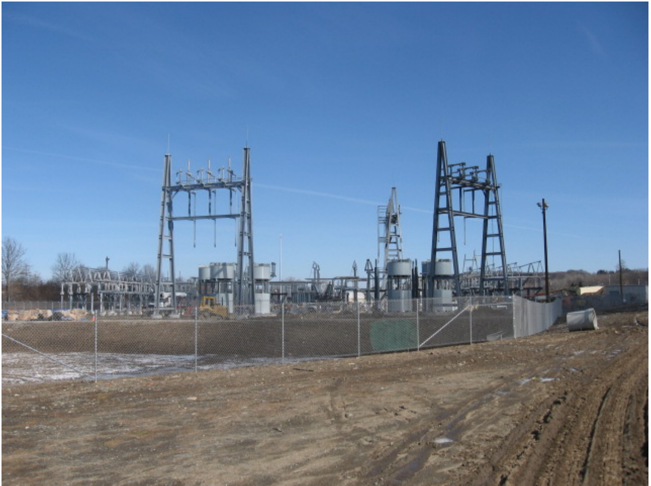
East Devon Subststion (Milford): A general view of construction at the substation.
