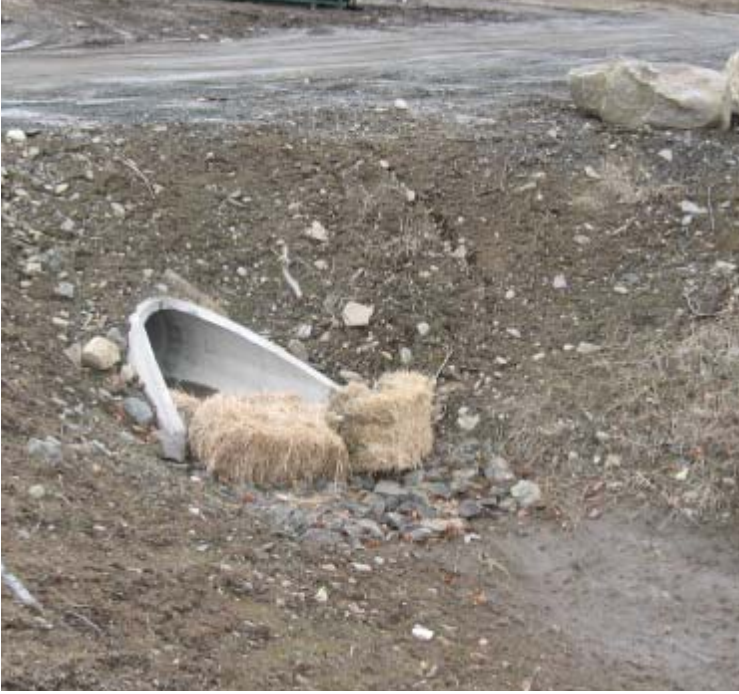
East Devon Substion (Milford): Haybale controls have been installed at a culvert outlet within the drainage swale located along the eastern boundary of the substation.
