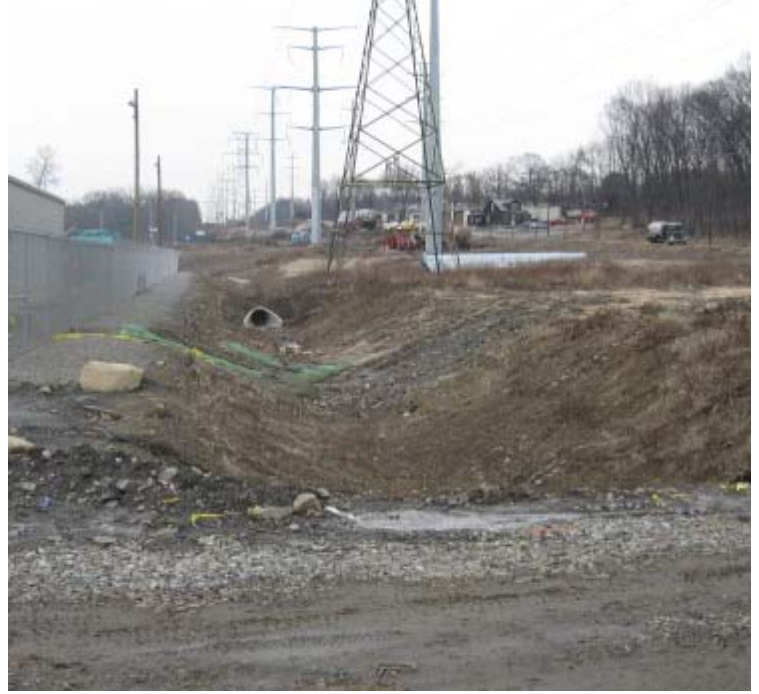
East Devon Substation: Exposed soils have been temporarily stabilized with mulch within the drainage swale.
