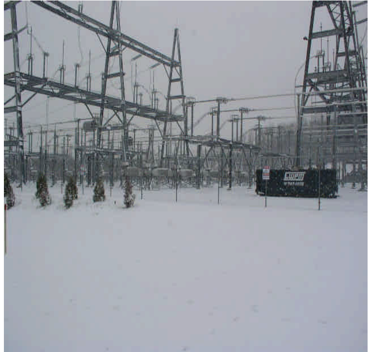
View of the switching station looking from the east to the west.
