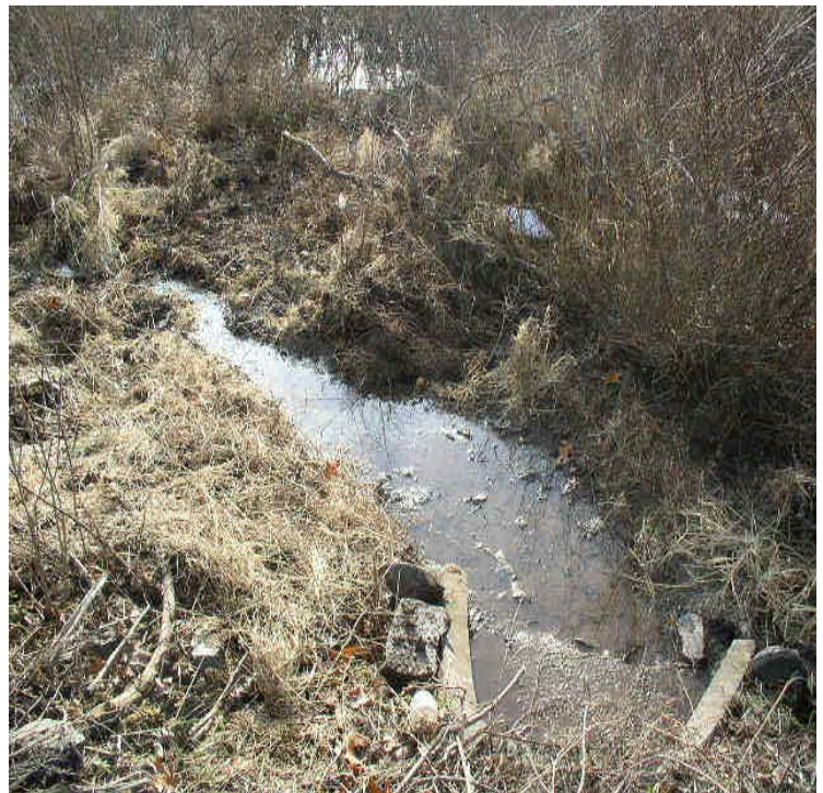
Accumulated sediment has been removed from the wetlands and culvert. Mulch was placed over exposed areas to reduce possible erosion or run-off.
