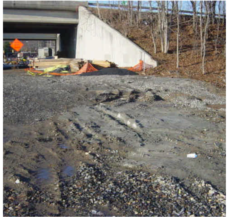
Concrete washout remains near sta. #15 along the shoulder of the roadway. Ruts through this area appear to be recent and therefore due to other vehicles, since work has shut down for two weeks.
