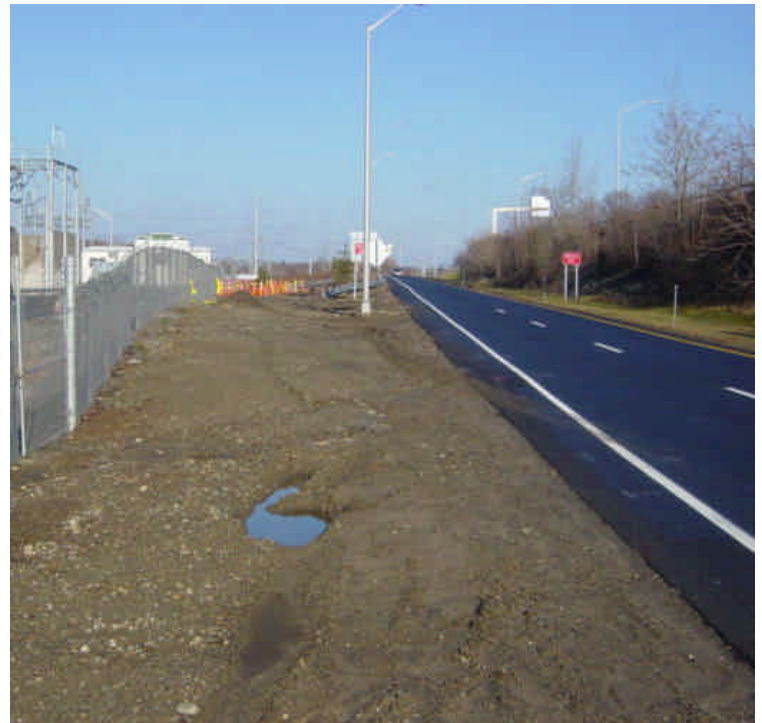
Trenching will continue in the area of sta # 5-7 near the Rt. 7 off-ramp. Portions have been backfilled. The contractor stated that they would reestablish the pre-construction drainage swale once work is complete in this area.
