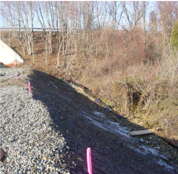
View of the slope near sta #15 (vault #1) The silt fence here was still overtopped with stone and needs repair. A concrete washout was also observed along the slope with run-off to the silt fence. The concrete washout needs to be removed and future washouts need to be properly contained.
