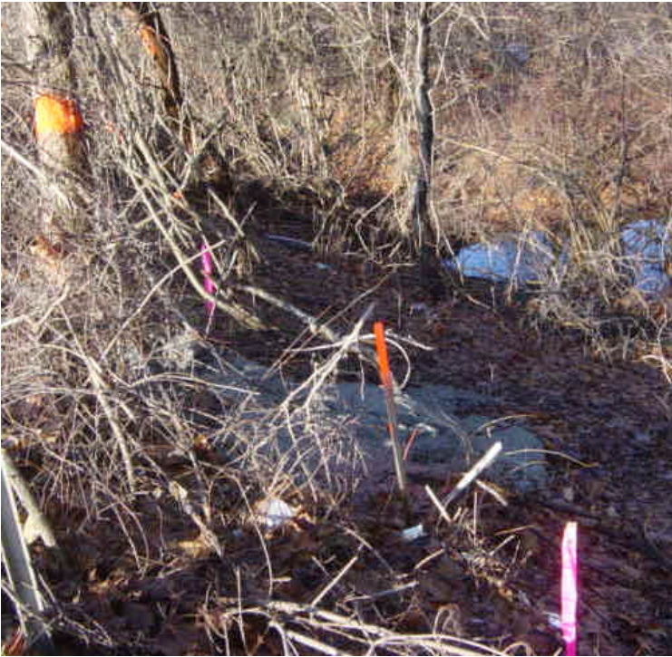
A concrete washout remains on the slope near the work at sta. #16-18. Haybales have not been reset and there are no controls between the work and what appears to be a resource area down-gradient. Trees were marked for removal in this area.
