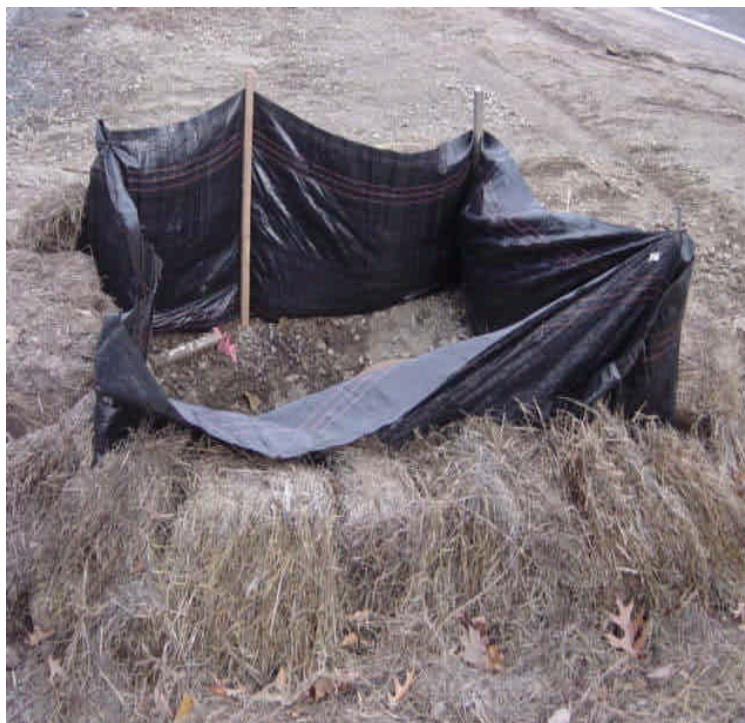
Drainage inlet near sta. #9+50 has been protected with silt fence and haybales, however accumulated sediment remains. The structure was associated with a pre-construction drainage swale which was not re-established after trenchwork altered the area. Efforts need to be made to ensure appropriate drainage.
