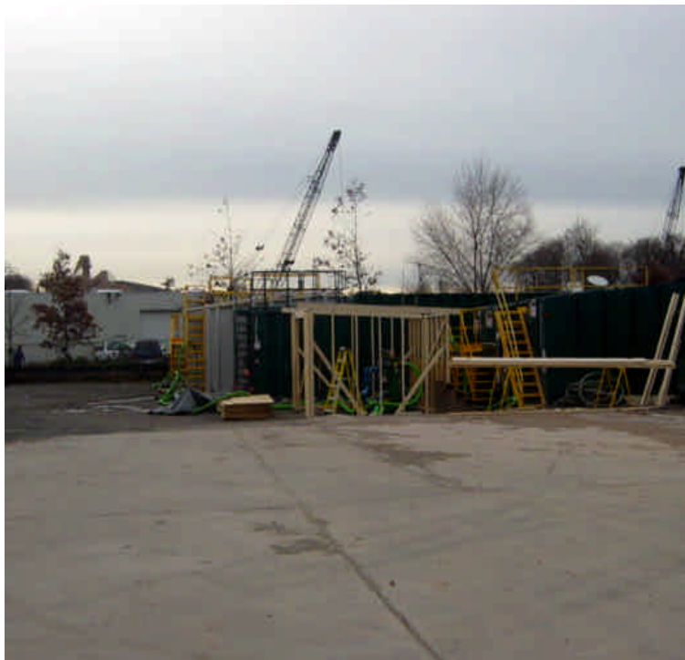
Contractor lay-down yard located on Smith Street in Norwalk is primarily being used to store frac tanks. No equipment or materials are being stored in the yard at this time.
