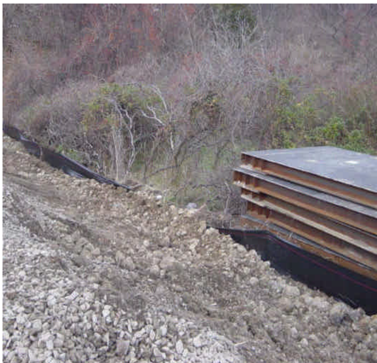
Silt fence has been proactively installed along the base of the slope near sta. #15-16. In several places, the soil/stone had piled up and was overtopping the fence. Plates were also being stored beyond the barrier.
